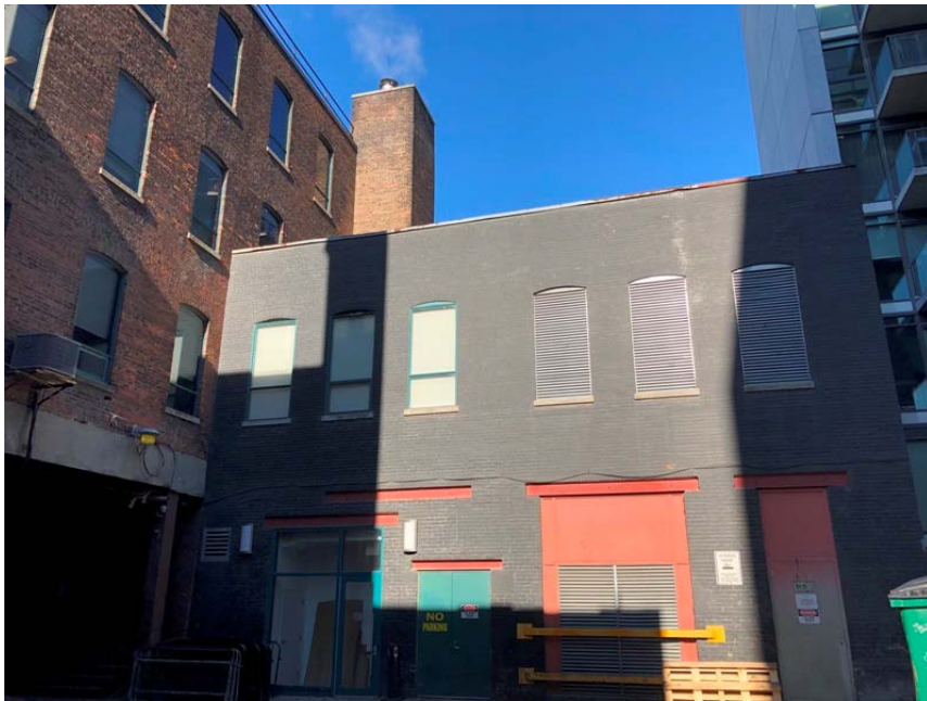
33. 473 Adelaide Street West, rear (south) elevation of the two-storey wing facing the laneway, with later modifications showing the original steel lintels, with the side (east) elevation of the four storey main building to the left (HPS, 2020)
