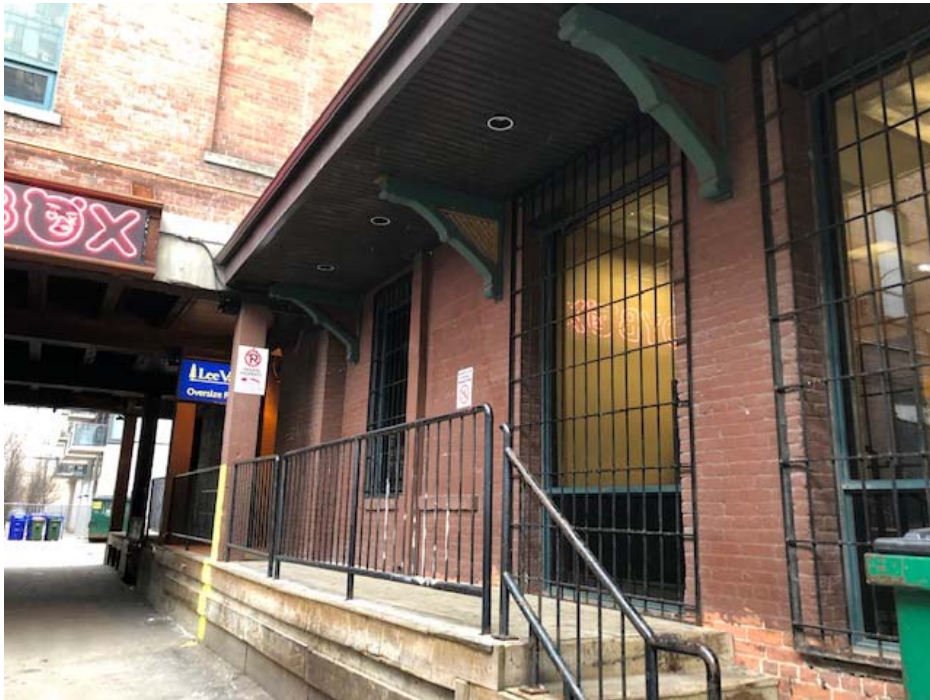
32. 582 King Street West, loading dock at the north elevation of 588-592 King Street West (HPS, 2020)
