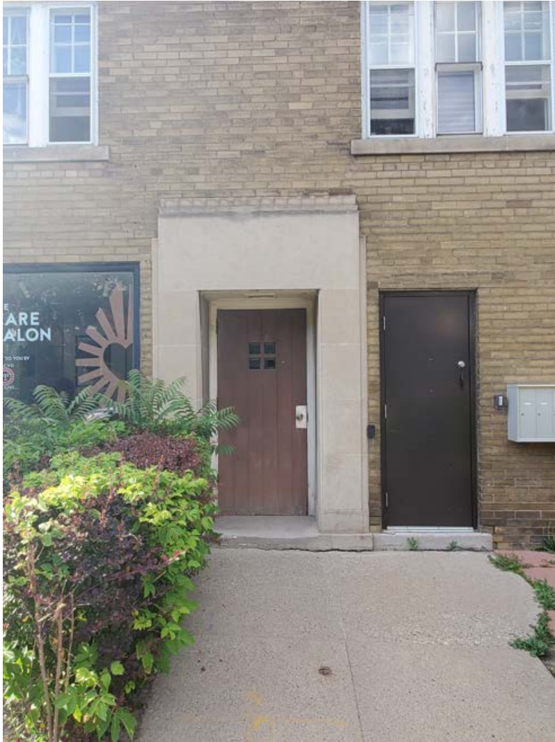
11. Detail of the recessed entrance set in the decorative stone surround in the side (south) elevation (Heritage Planning [HP] Photo)
