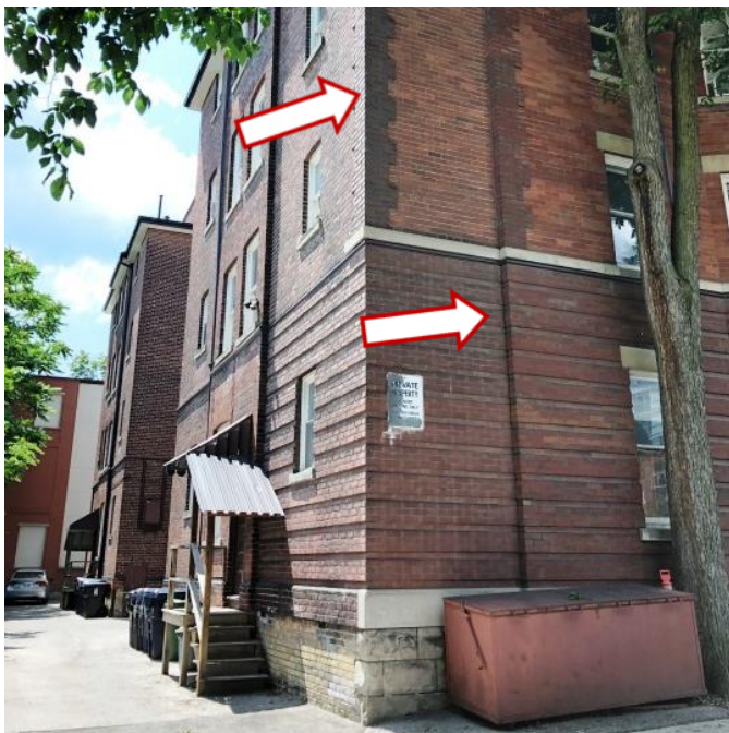
27. Rear, east elevation showing the later bathroom addition as indicated by the different colour of the purple brick especially evident in the quoins and in the jog in the wall between the enclosed stair and the two adjacent bathroom volumes. (HP, 2019)
