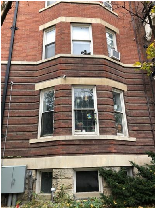
23. Photograph of one of the bay windows on the west elevation showing the materials including the rough-hewn stone blocks, Roman stone bands and lintels, purple bricks of the rusticated base and the red brick of the upper stories (HP, 2020)
