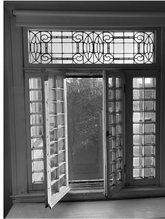
An example of one of the leaded glass and casement windows in the dining rooms facing the courtyards
