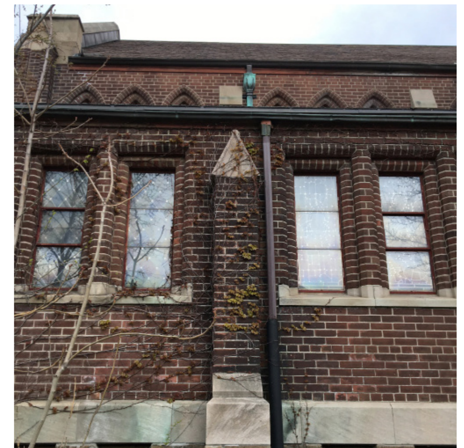
South elevation showing vine growth and damage; and missing windows - typical (ERA, 2020).
