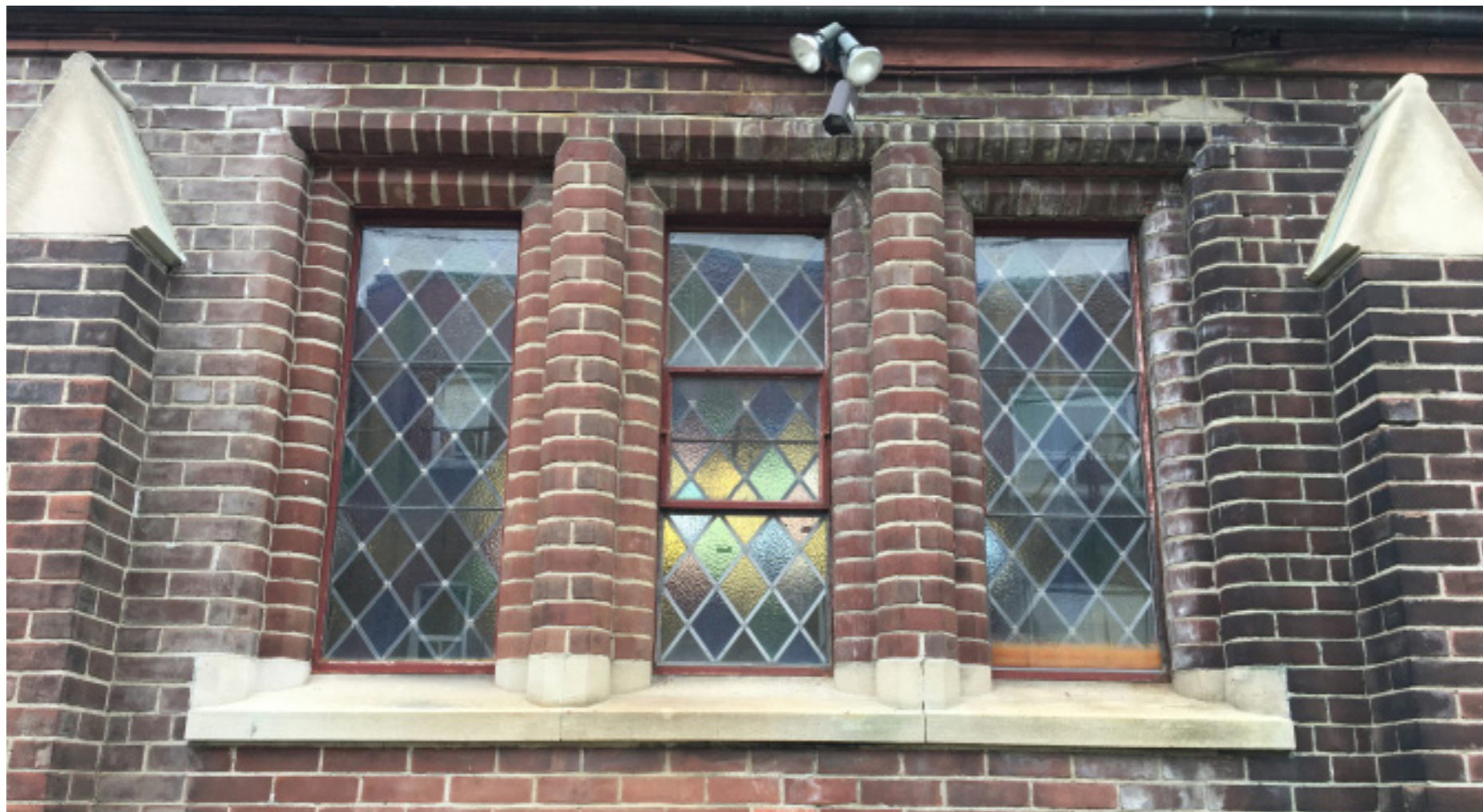
North elevation showing spalling brick, environmental staining, efflorescence, face brick erosion from clinging vines and miscellaneous ferrous metal penetrations/services on the exterior of the building - typical (ERA, 2020)
