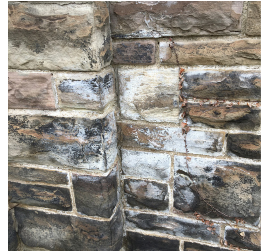
Efflorescence on ashlar base - typical (ERA, 2020).
