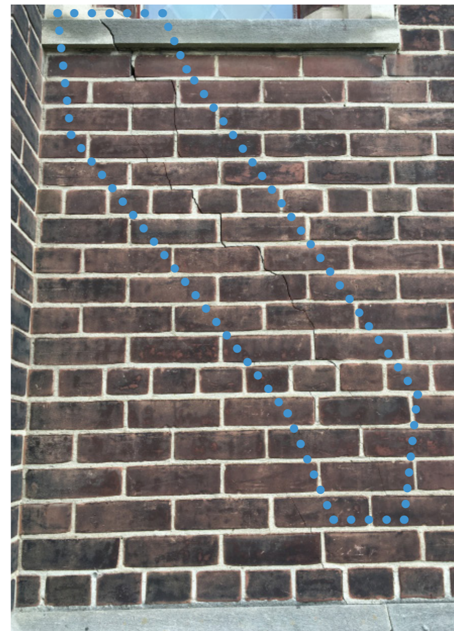
Step crack through masonry and sill (ERA, 2020).
