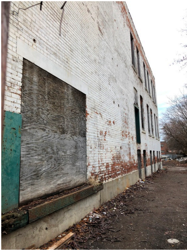
27. Side (west) elevation showing the loading bay and the pairs of window openings (HPS, 2020)
