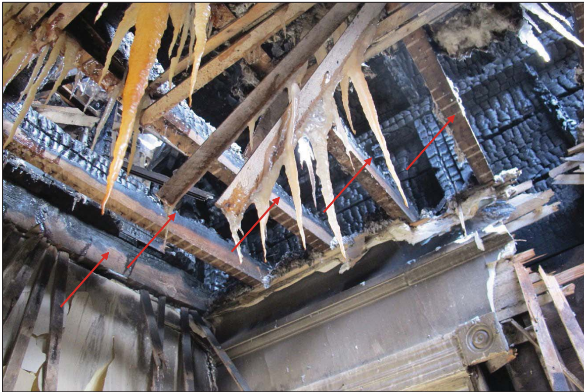
Figure 14: View of charred floor joists above second level kitchen
