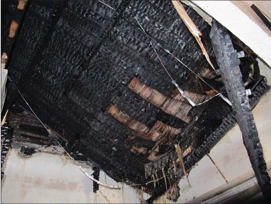
Figure 12: View of collapsed portion of second floor level in northeast corner
