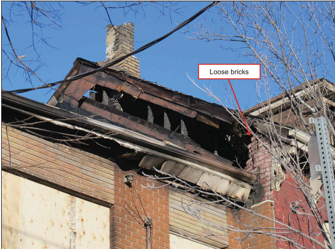
Figure 5: View of subject building showing cracked facade with loose masonry bricks
