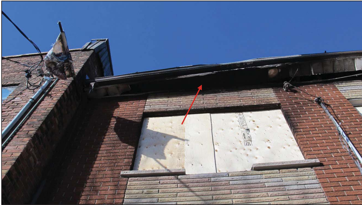
Figure 3: View of east elevation of 160 Bathurst Street showing blackened roof soffit
