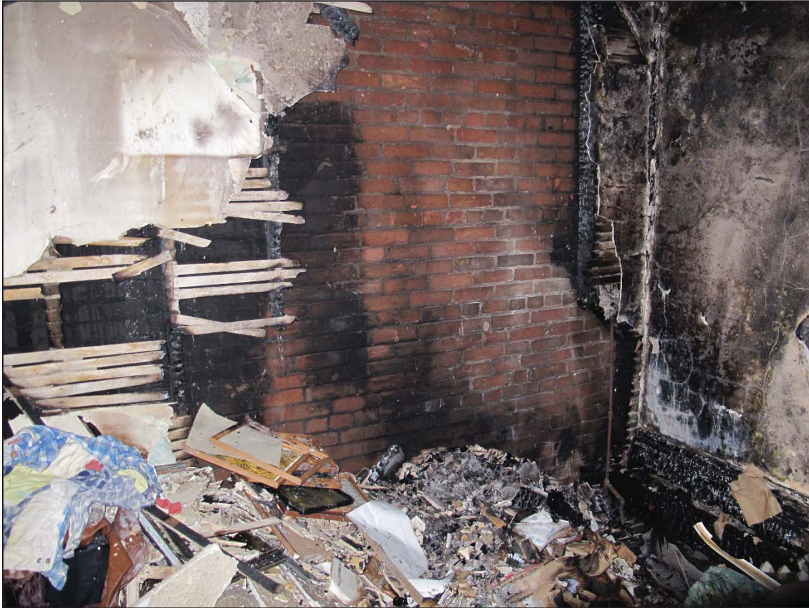
Figure 15: View of north wall at second level showing burnt wood studs and blackened neighbouring masonry wall
