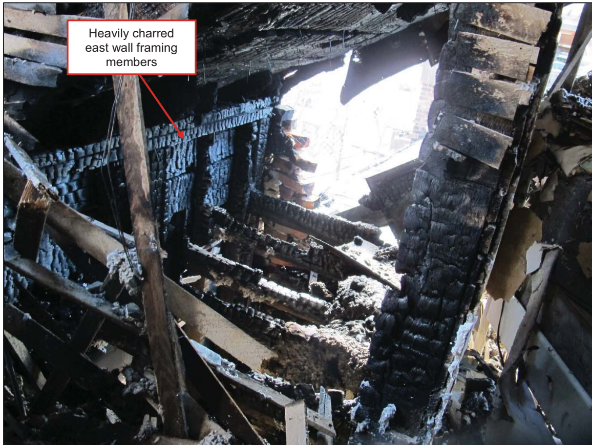
Figure 17: View of southeast corner of third level showing fire damaged framing members
