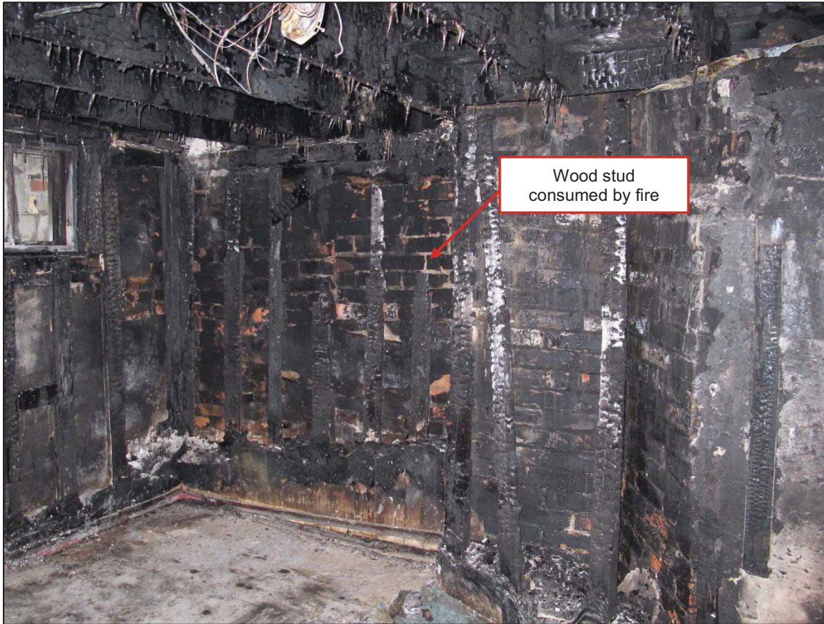
Figure 7: View of east end of south wall in basement showing charred wood studs and wall framing
