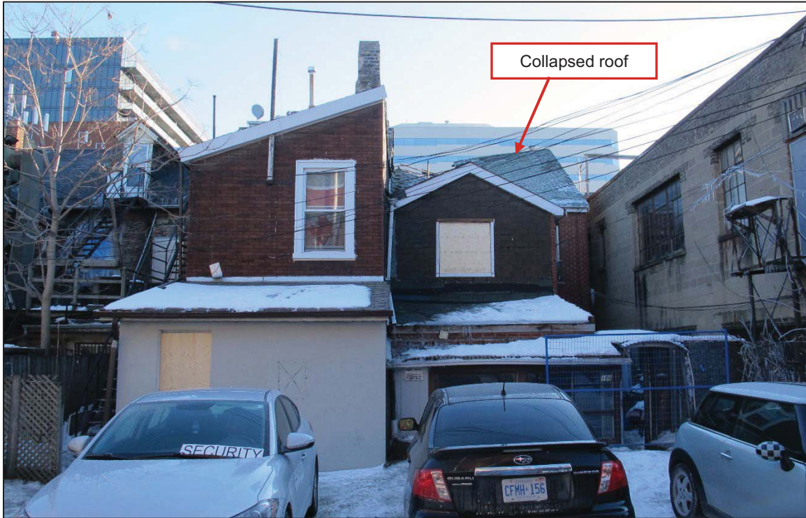
Figure 2: View of west elevation of subject building showing collapsed roof at 160 Bathurst Street
