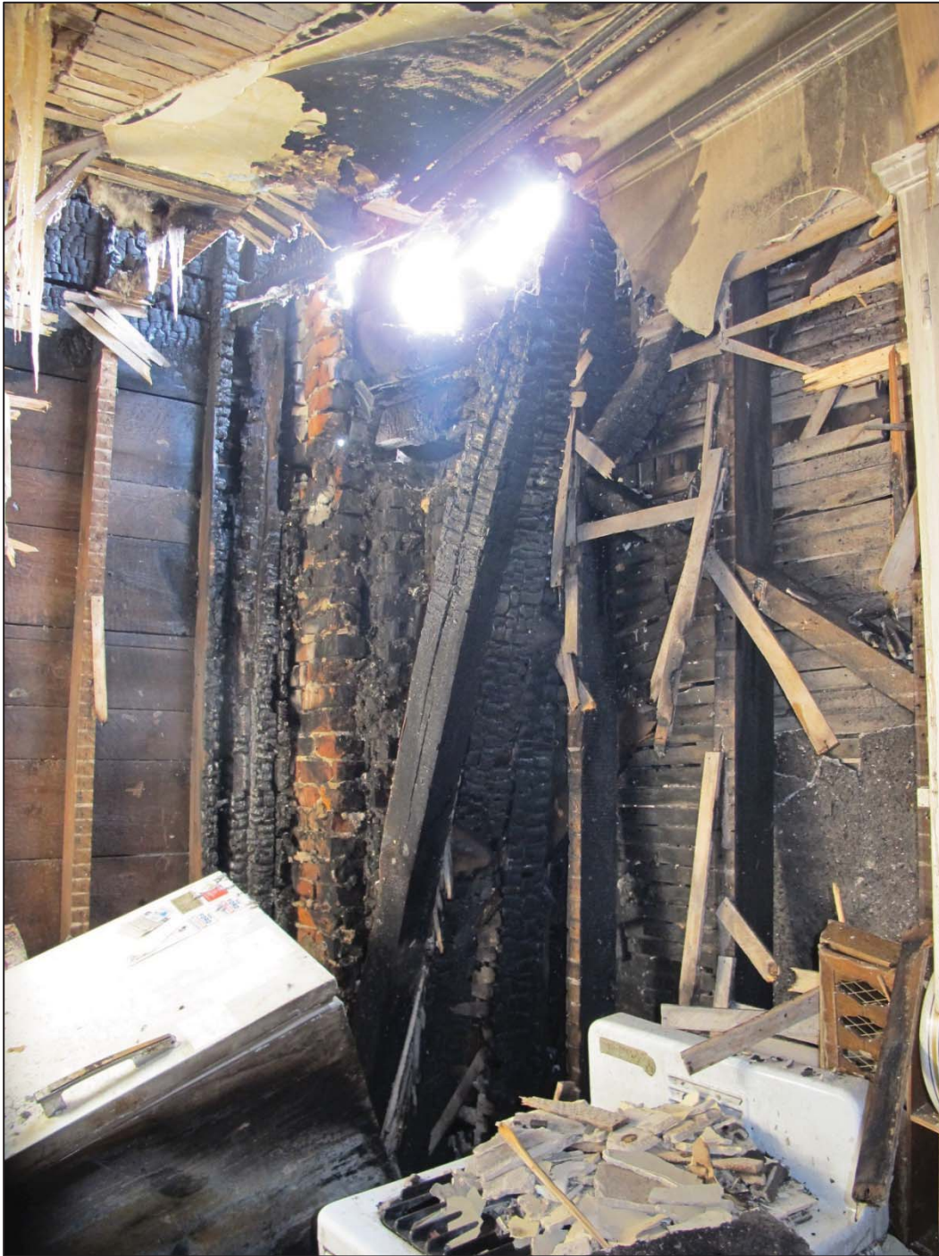
Figure 13: View of south party wall at second level showing fire damaged wood studs
