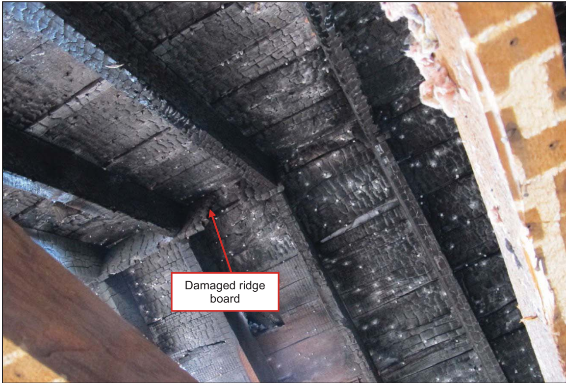
Figure 16: View of roof structure showing burnt rafters and partially consumed ridge board
