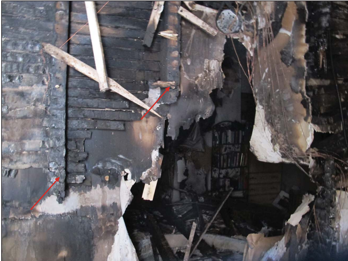
Figure 9: View of fire damaged studs in loadbearing wall on ground level
