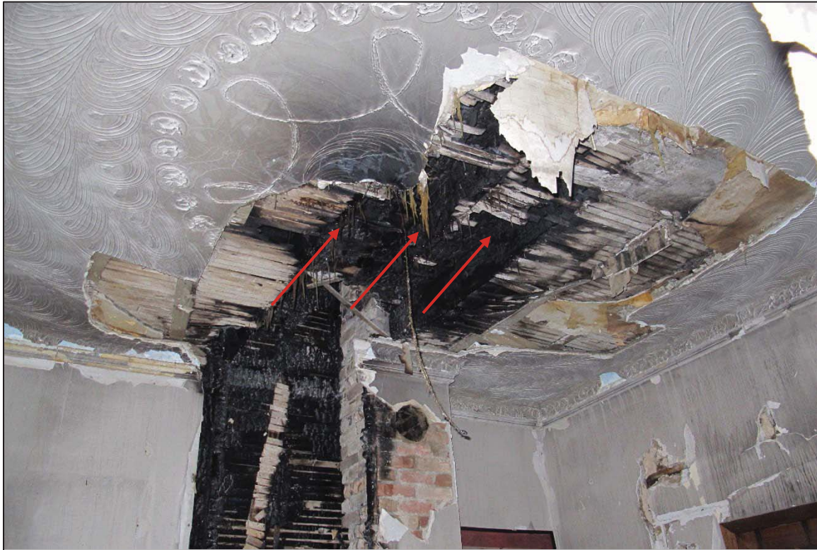
Figure 8: View of charring on second level joists above southeast ground level bedroom
