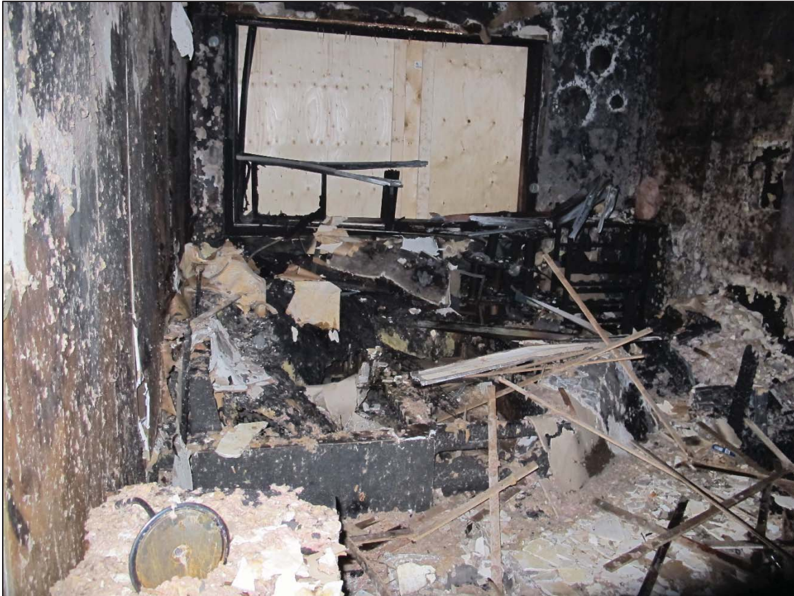
Figure 11: View of southeast room at second level showing extensive smoke and soot damage
