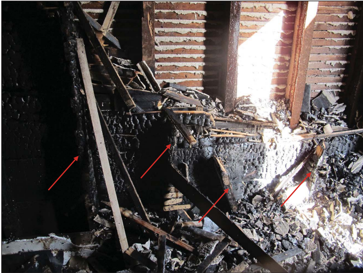
Figure 10: View of fire damaged studs in north wall on ground level
