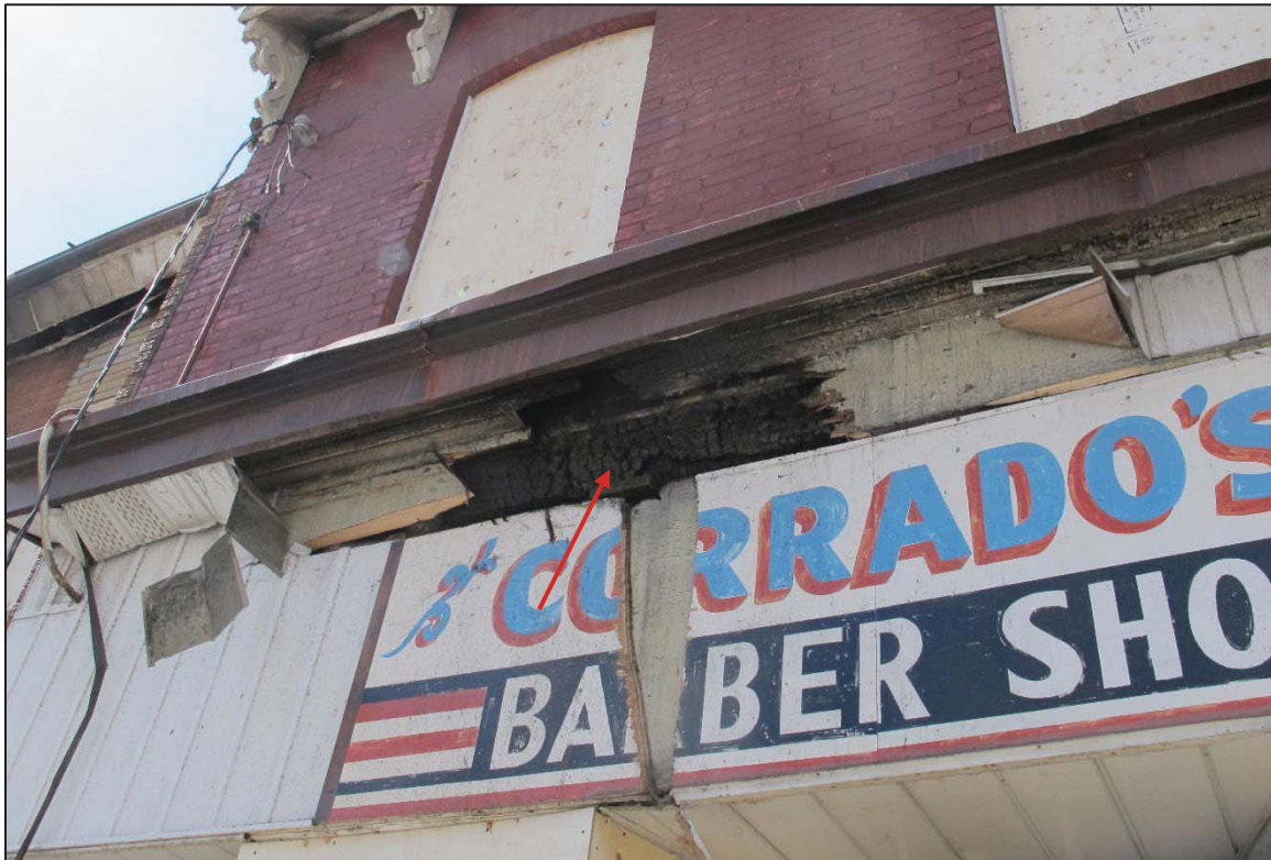
Figure 4: View of east elevation of 162 Bathurst Street showing fire damaged soffit and fascia
