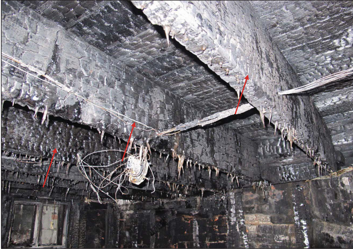
Figure 6: View of ground floor framing in southeast bedroom showing extensive fire damage and charring to wood decking and wood joists
