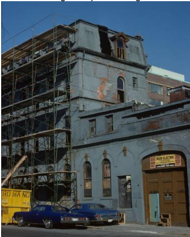
14. 1978 Photograph taken during the restoration of the elevations of the Little York Hotel and showing the west elevation of the Stables and Coach house at 65 George Street prior to restoration/alterations. (CTA Fonds 1526, File 51, Item 5)
