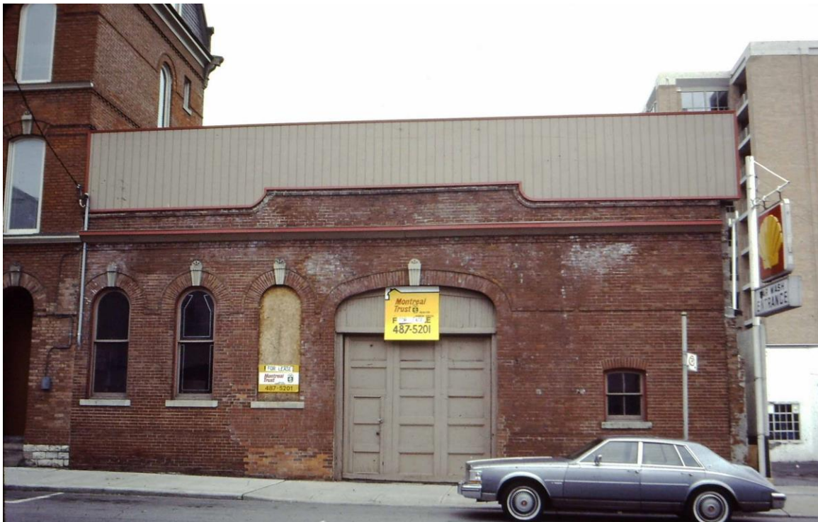
16. 1983 Photograph of the hotel and stables building following the restoration of the principle (west) elevation of the stables. The photograph shows the restoration of the brick, the restoration of the original window opening with the removal of the doorway next to the carriage way and the alteration to the second floor elevation behind the brick parapet (THB - CTA)
