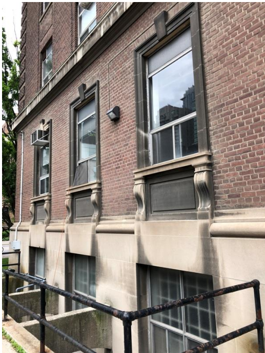
26. East (side) elevation, raised basement and ground floor, showing the stone cladding and classical details of the raised basement and stone surrounds with panels and keystones of the first floor windows with the projecting stone band between the first and second floors (HPS, 2019)
