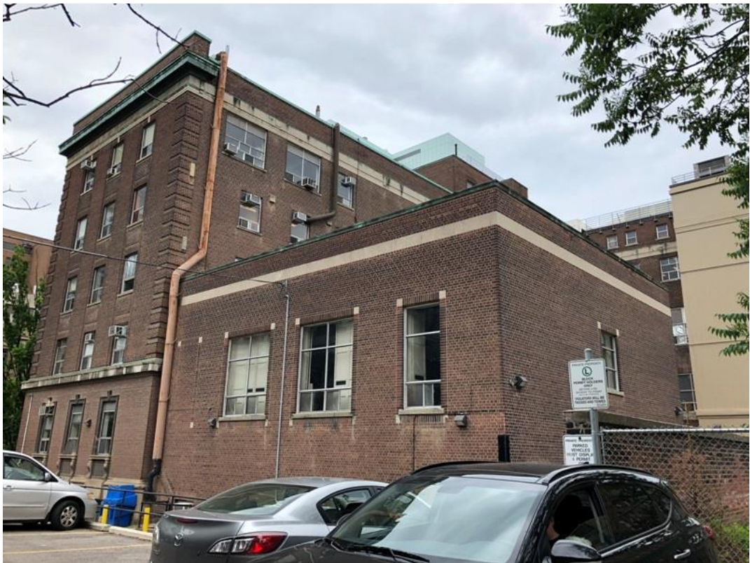
22. Banting Institute, east (side) elevation showing the end of the main block and the rear lecture hall (HPS, 2019)
