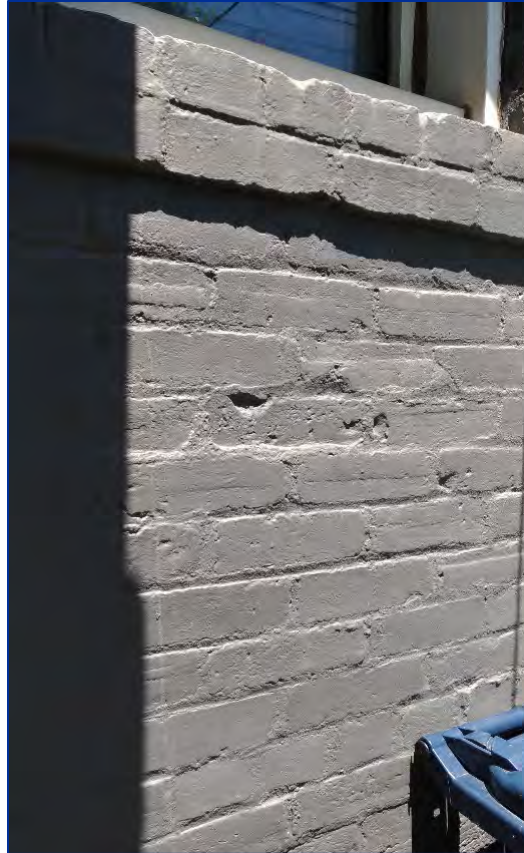
Figure 36: View of 44 Mitchell Avenue brick
