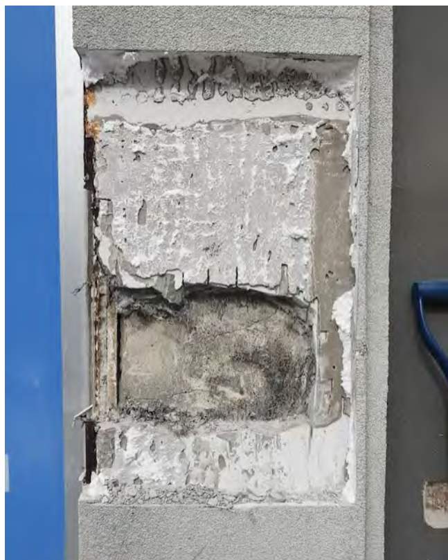
Opening near bottom portion of pilaster. The stucco was applied on a thick layer of expanded polystyrene, over what appears to be a stone panel. This panel was partly cut to reveal what appears to be a concrete pier.
