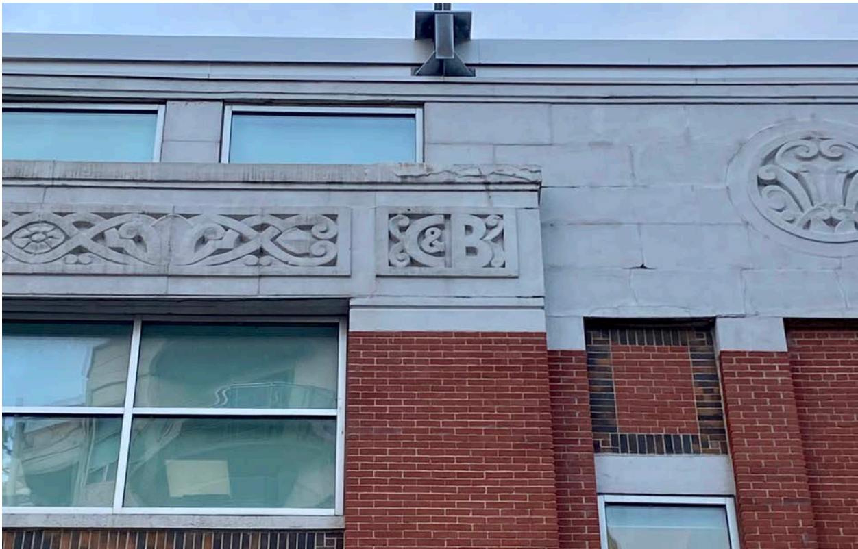
Figure 45: 545 Lake Shore Boulevard West; details of the building's east elevation, including decorative cast-stone motifs and the initials of Crosse & Blackwell. (Heritage Planning, 2021.)
