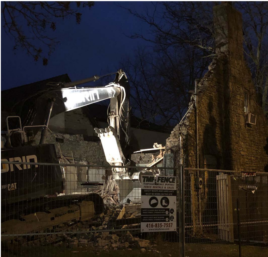
12. Complete demolition of the Frederic J.A. Davidson Cottage at 98 Superior Avenue by the owner on November 30, 2020, only hours before the property's consideration for designation by the Toronto Preservation Board. (Heritage Planning, 2020)
