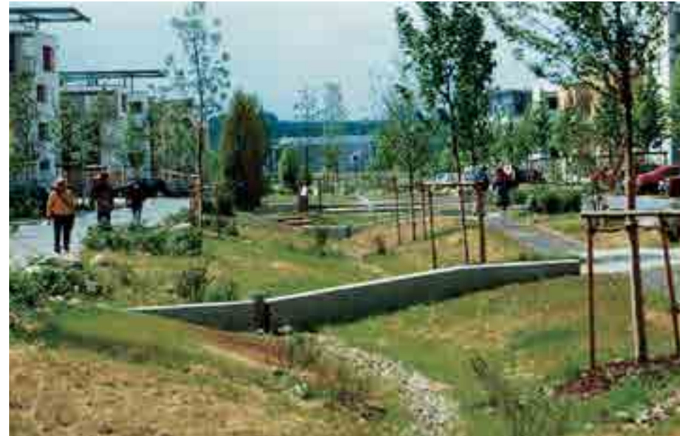
Figure 146. Landscape drainage solutions (Vancouver, Canada)
