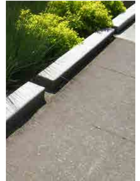
Figure 265. Bioswale inlets, Portland OR (image credit Jill Bliss)
