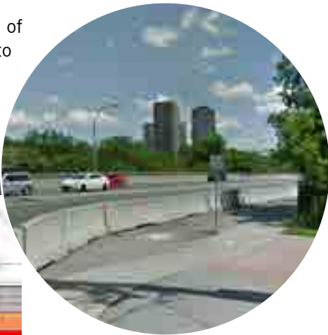
Figure 329. Existing jersey barrier condition along the Humber Bridge for pedestrians and cyclists
