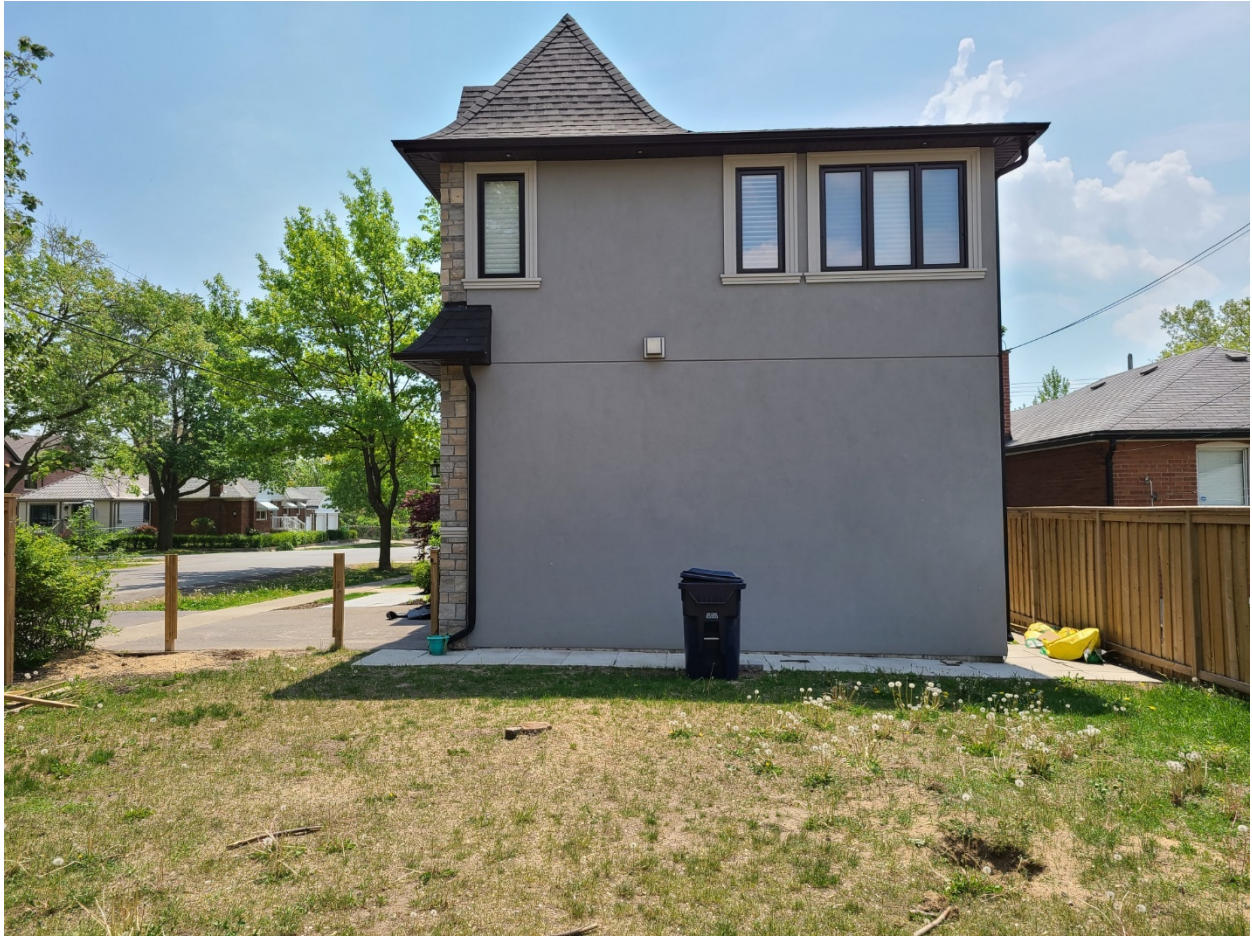
Attachment 2: photo indicates the garage used as part of the enclosure for the pool (photo taken facing South)
