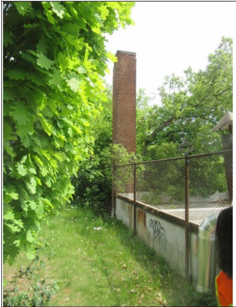
PHOTO NUMBER 7: North exterior wall at east end. Adjacent grade is near elevation of roof of building
