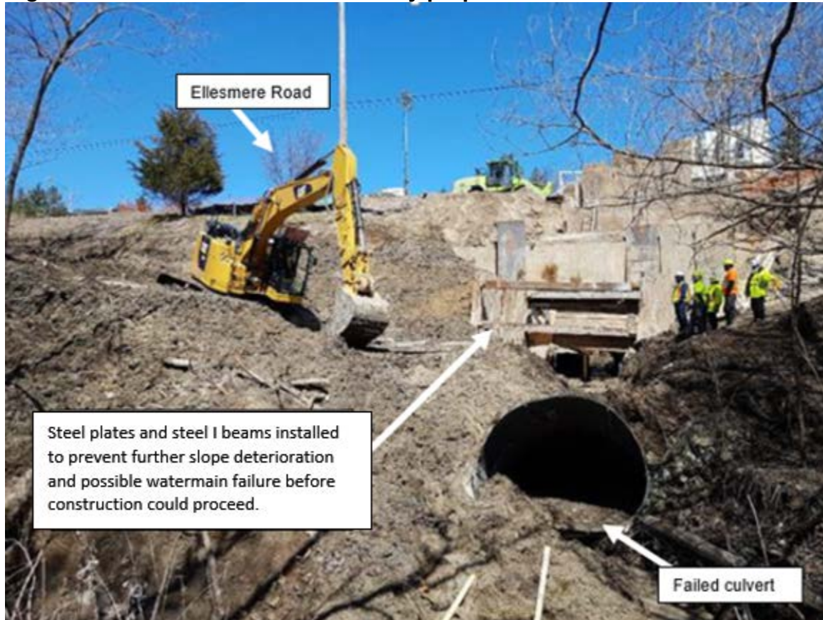
Figure 2: Failed culvert and site safety preparation
