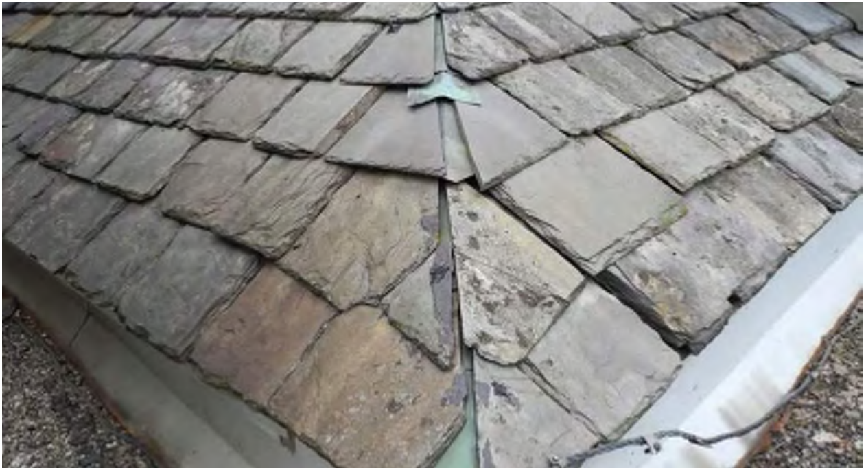
Figure 28: Detail of roof slates on northeast hip on the service garage showing cracked units, chipped edges and surface delamination ( CBCollective, 2019 ).
