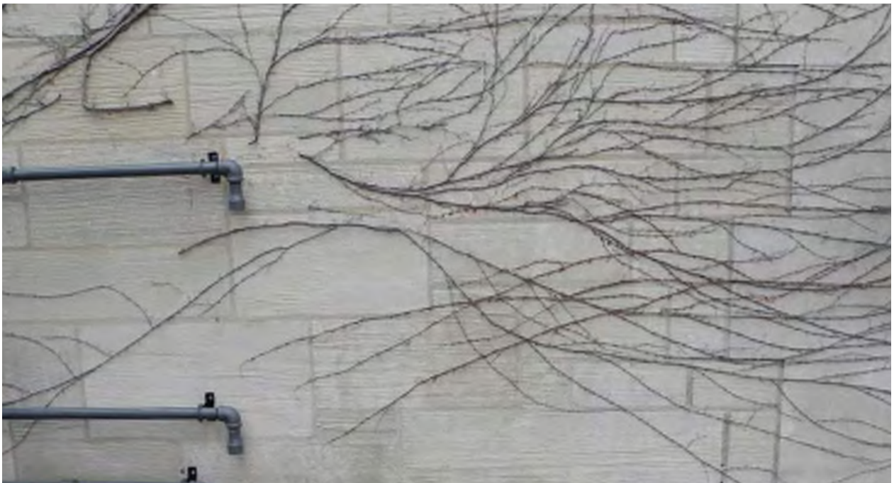
Figure 19: Detail of limestone masonry on the west elevation of the service garage, showing coursing, pointing and surface texture of the masonry (CBCollective, 2019).
