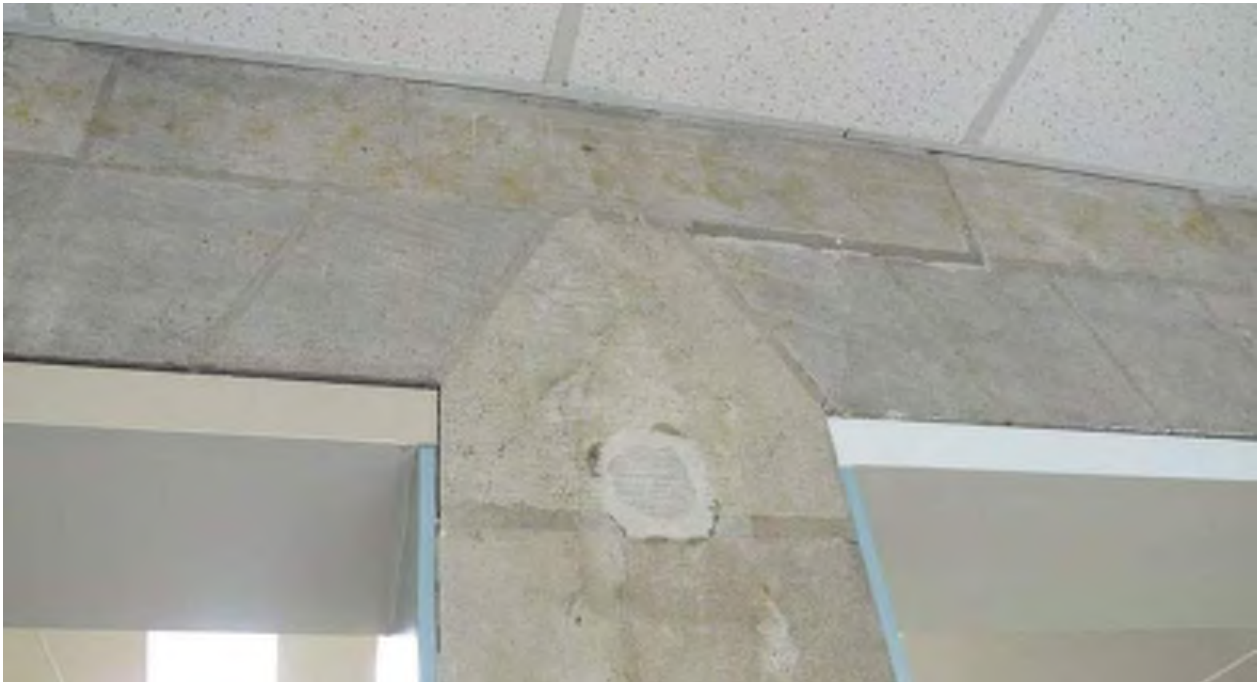
Figure 22: Portions of the original service garage south elevation remain visible inside the addition (CBCollective, 2019).
