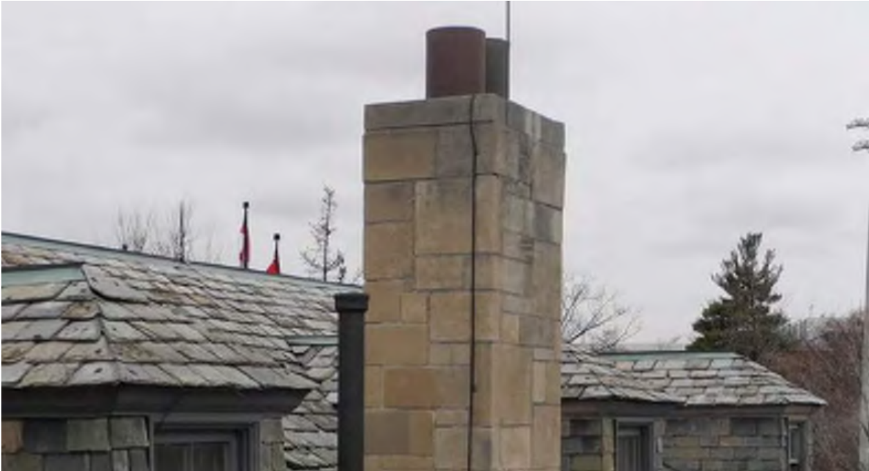
Figure 21: Detail of the service garage chimney, showing conditions of deterioration nearer the top (CBCollective, 2019).
