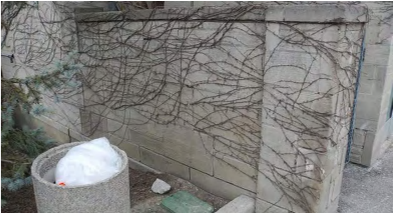
Figure 20: Landscape wall at the southwest corner of the service garage. Efflorescence, mortar loss, and displacing masonry units are apparent (CBCollective, 2019).
