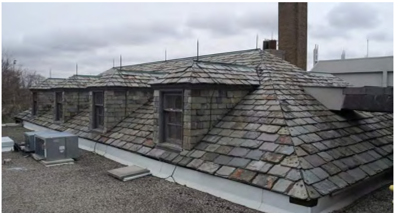
Figure 17: Roof dormers on the south side of the service garage, have been severed from their original relationship to the historic south elevation (CBCollective, 2019).
