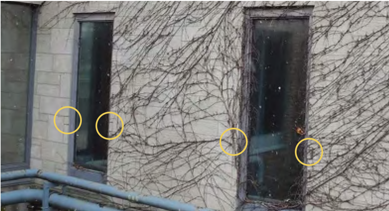
Figure 24: Altered window openings on the unobstructed portion of the service garage’s north elevation. Remnants of the original stone sills can still be observed, highlighted by yellow circles (CBCollective, 2019).
