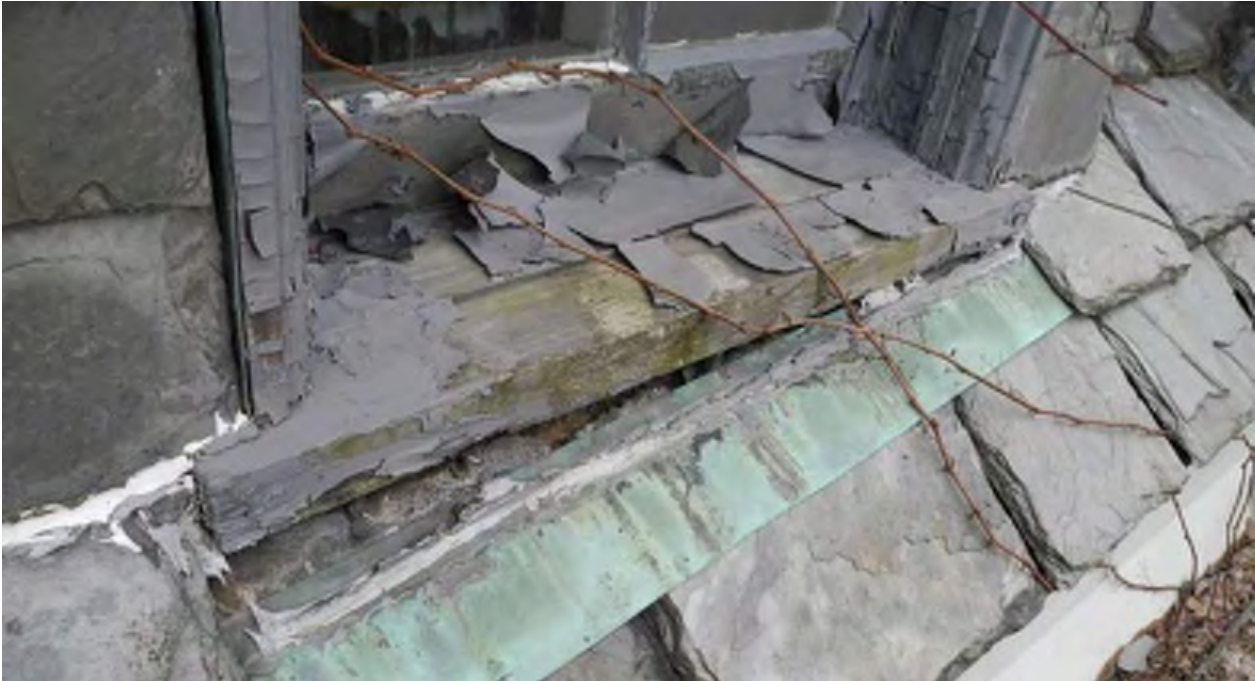
Figure 25: Paint failure and rot as observed on a dormer at the service garage’s north elevation. Note displacement of the flashing below as well (CBCollective, 2019).
