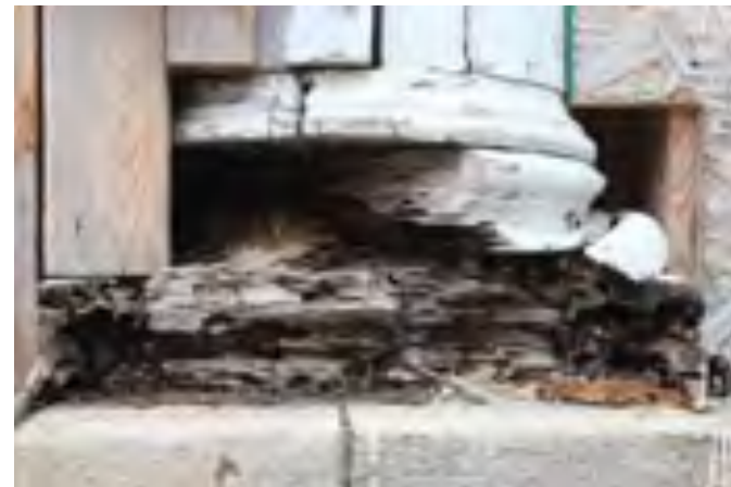
Wood rot at column base
