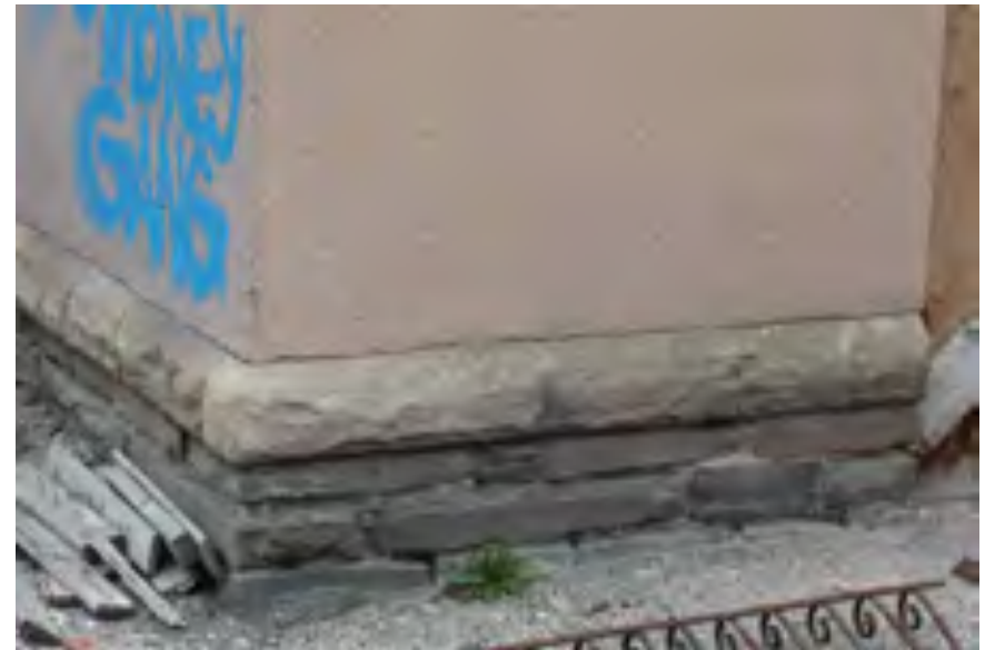
Rubble stone used along the water table of the rear addition walls
