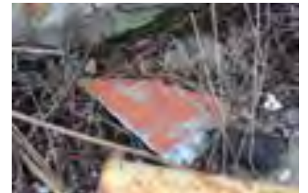
Damaged piece of stucco with brick face bonded
