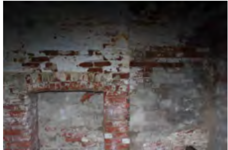
Masonry foundation wall along south facade. Note the parking, painted bricks, efflorescence buildup and fireplace
