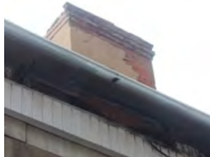
North chimney note the loose bricks, damaged stucco and bricks
