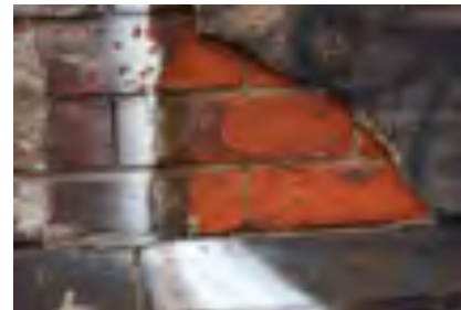
Damaged brick face under stucco
