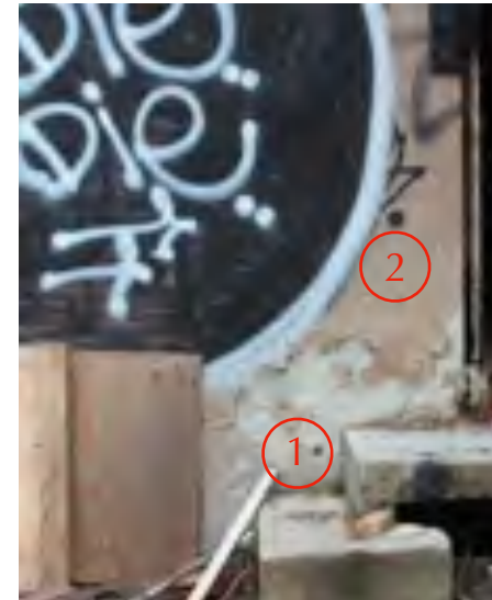
Typical stucco rendering over brick note the cement parging base (1) and pink textured rendering (2).
