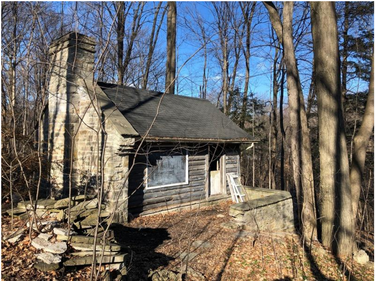
50. West and south elevations of the cabin showing the combination of west stone wall with chimney and log walls with stone terrace walls
