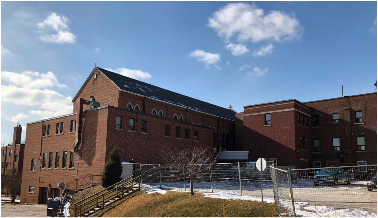
42. Rear south elevation showing the 1958-9 chapel with the sacristy-oratory volume wrapped around the west end, with the kitchen and garage at the lower levels and to the right the earlier wings of the seminary
