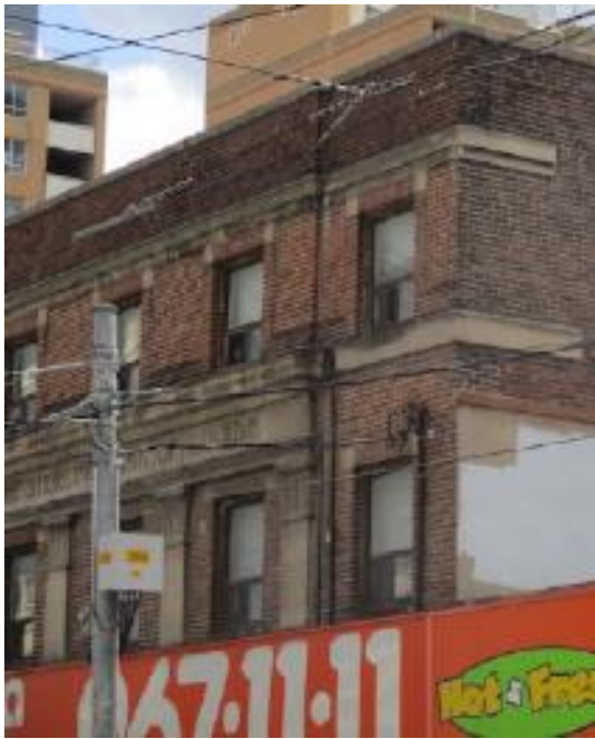
11. Current photograph showing the intentionally-designed return of the upper level stringcourses on the west elevation
