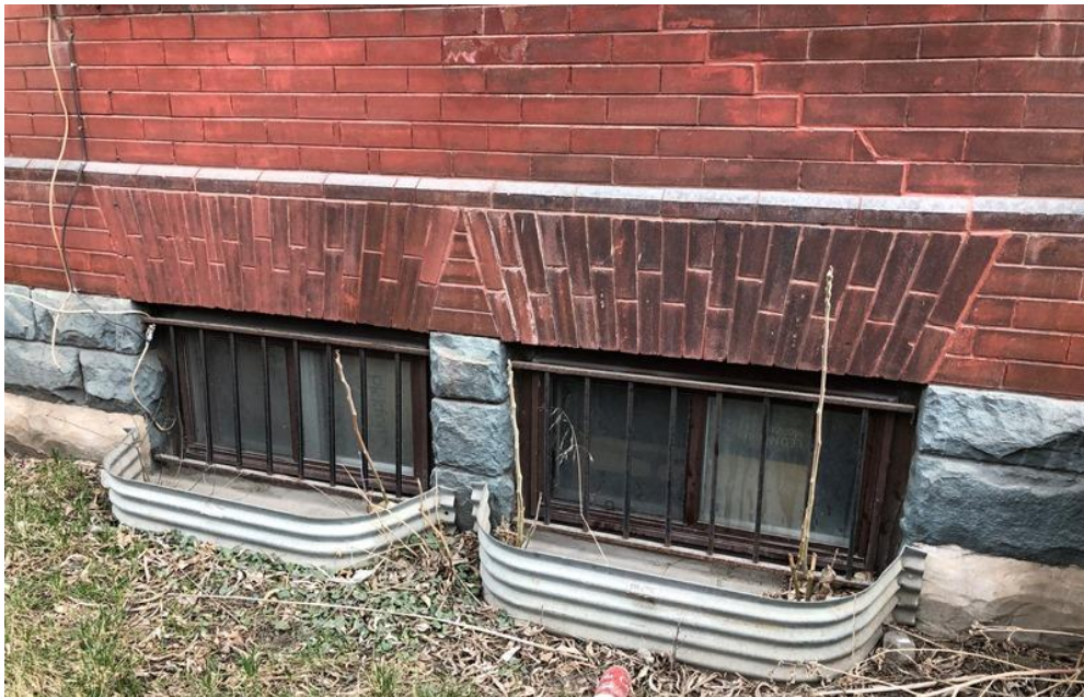
15. 685 Queen Street East, North Elevation, Detail of the stone foundation and the brick work: Photograph showing the details of the stone foundation and the brickwork on the principal, north elevation. Note the careful patterning and mortar joints of the paired basement windows (HP, 2021)
