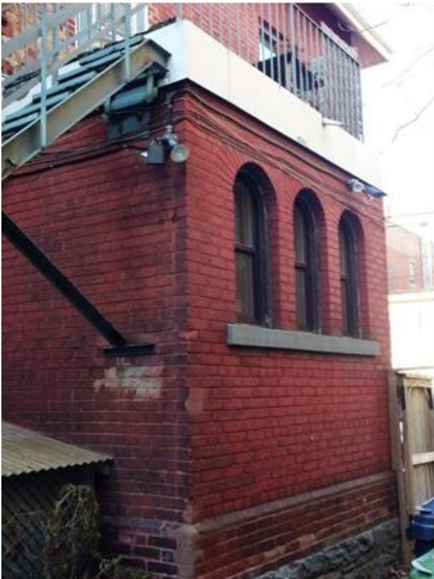
10. 685 Queen Street East, medical office entry porch, east elevation: Photograph showing the triple arched windows and continuous sill of the side entry porch and the brick details at the base. (HP, 2015)
