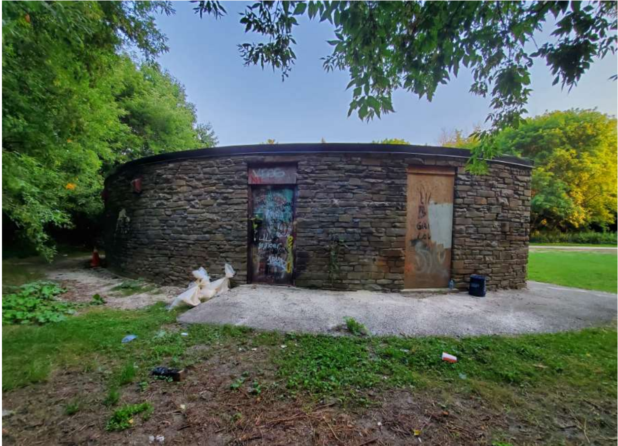
Figure 19. Detail of the men's washroom entrance in the rear (north) elevation (Heritage Planning, 2021)
