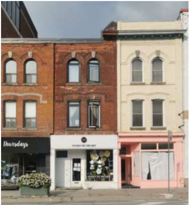
14. Current photograph of the principal (east) elevations of 1130-1134 Yonge showing the openings, the brick and stone detailing and the loss of the roof cornice and parapet at 1130 and 1132. (Heritage Planning, 2021)
