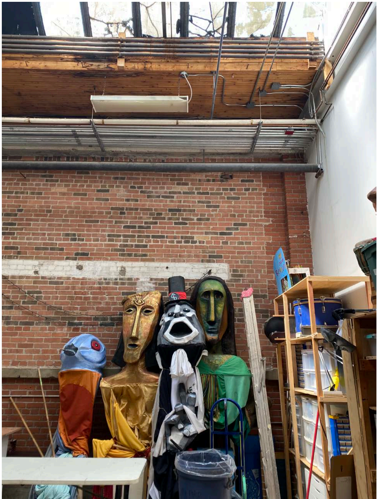
Figure 48: Interior of a unit within the subject property's southern portion, showing high ceiling and skylight; currently used by a theatre company. (Heritage Planning, 2021.)
