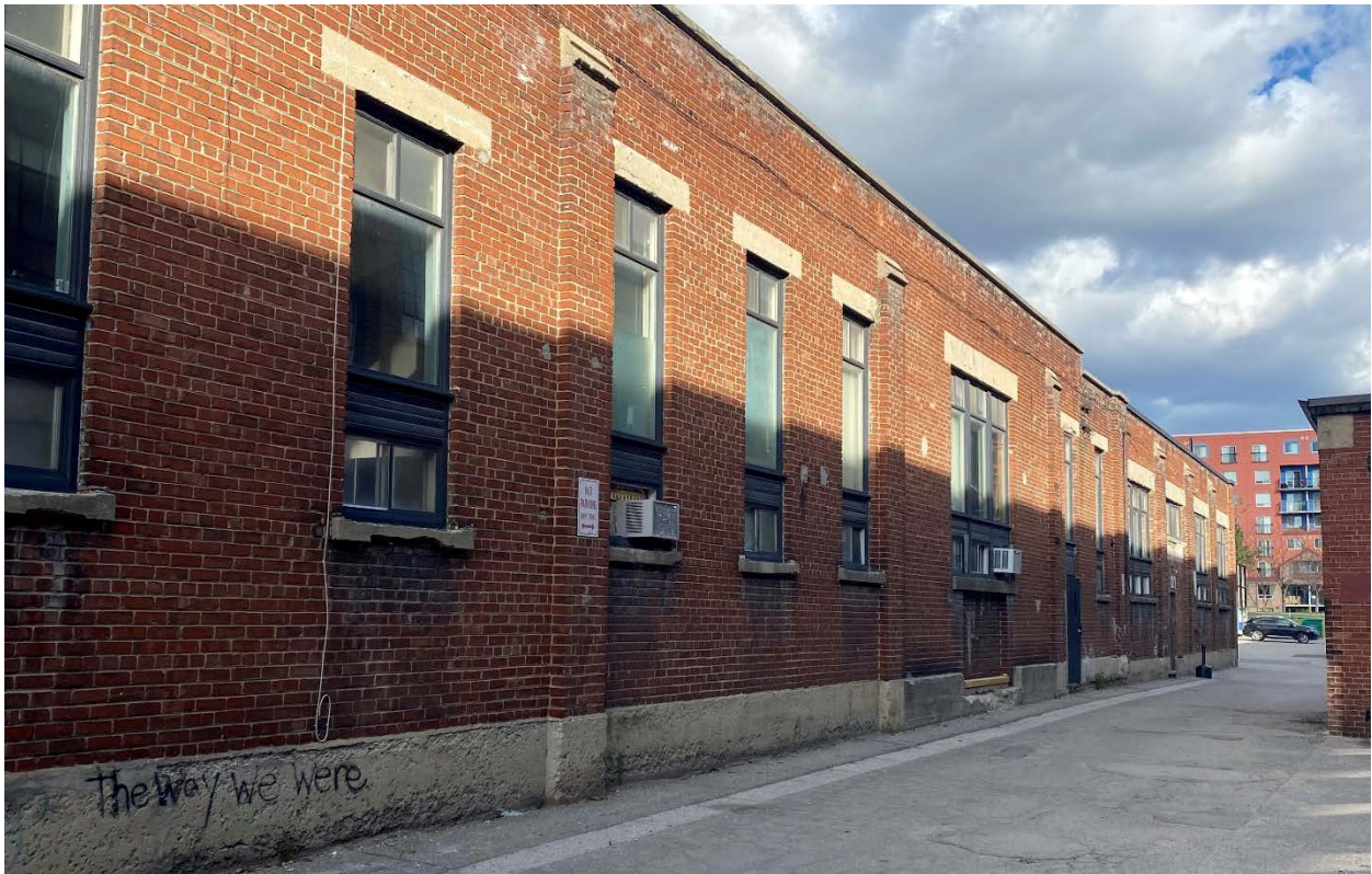
Figure 30: Northeastward view of the subject property's south elevation (dating to c.1914-1918). (Heritage Planning, 2021.)
