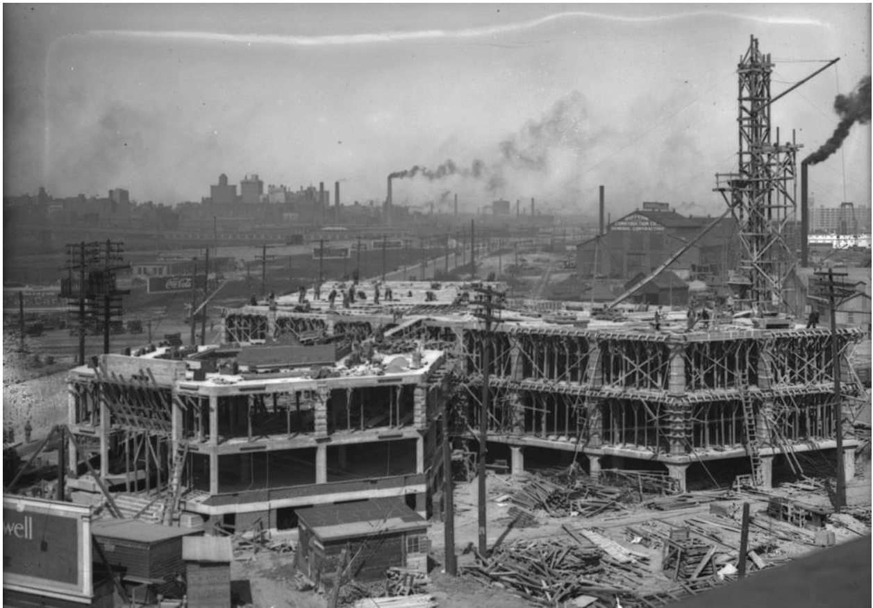
Figure 16: The subject property under construction, 1927. (Toronto Harbour Commissioners / Library and Archives Canada / PA-098619 – MIKAN 3656094 – 1927.)
