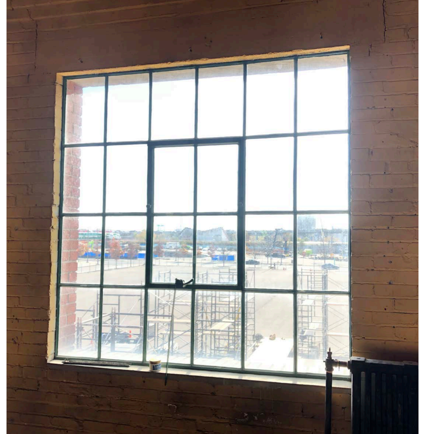
Steel window at warehouse to be rehabilitated. Photo from ERA
