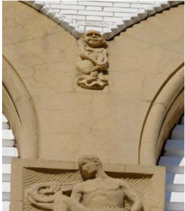
22. and 23. Details showing cast stonework by Merle Foster, whose work was both Classically-inspired (man with car and tire, at left) and Medieval (imp-like creature at the springing joint above, at right).
