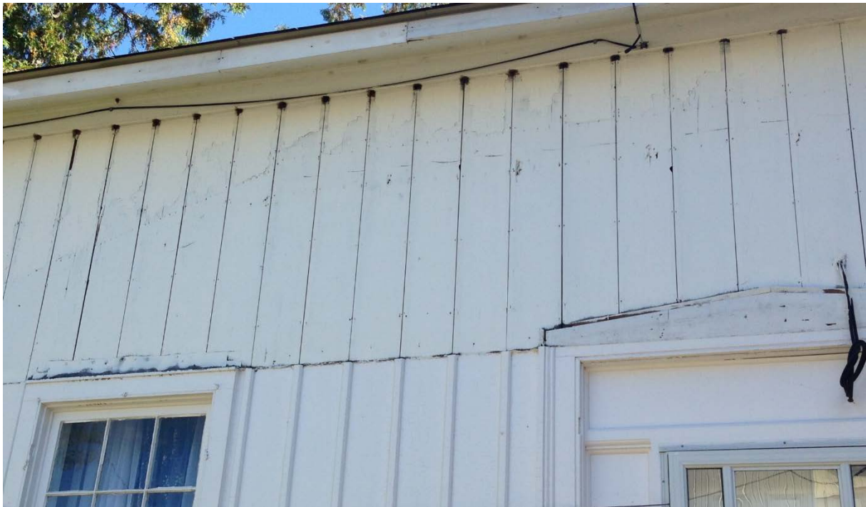
21. West elevation, showing the angled line of different paint indicating the roof line of the verandah and the missing board and battens above (HP, 2017)
