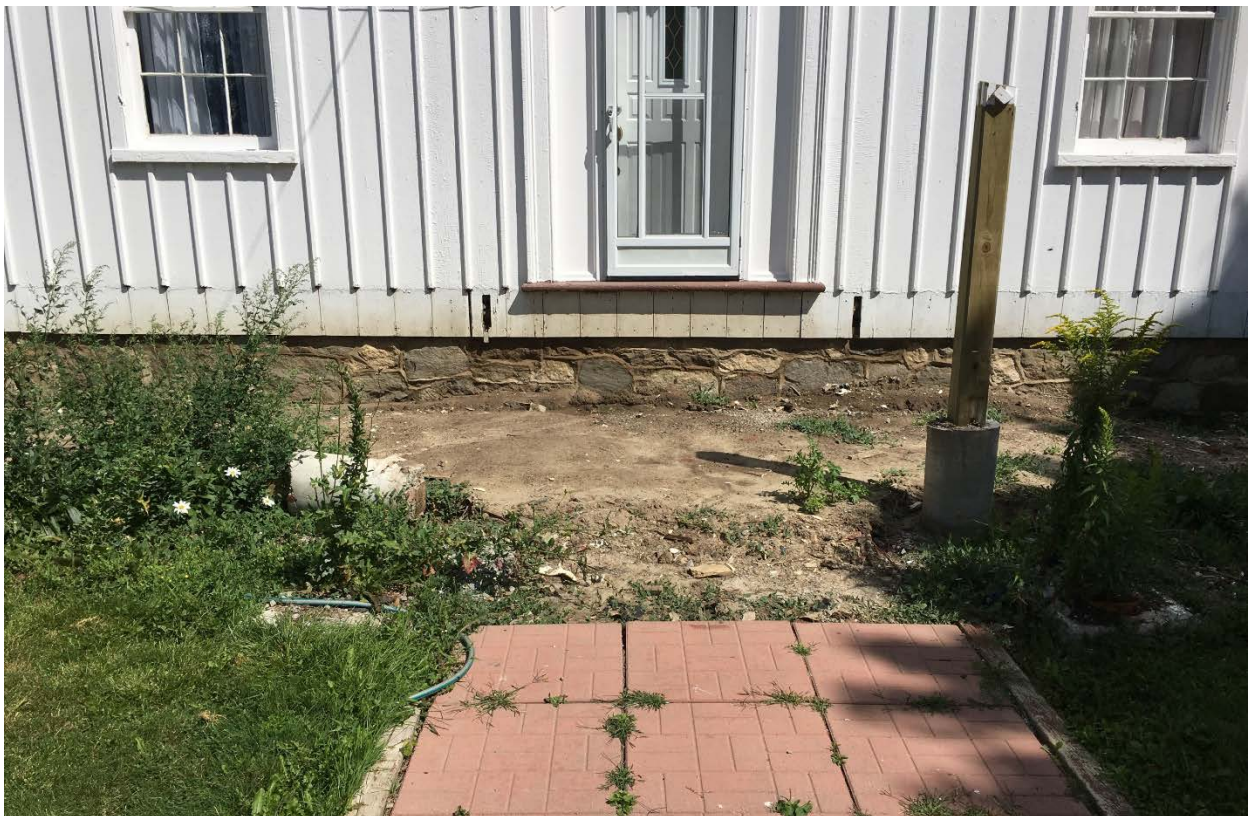
20. West elevation, showing the area where the verandah was located, and the path that lead to it (HP, 2017)
