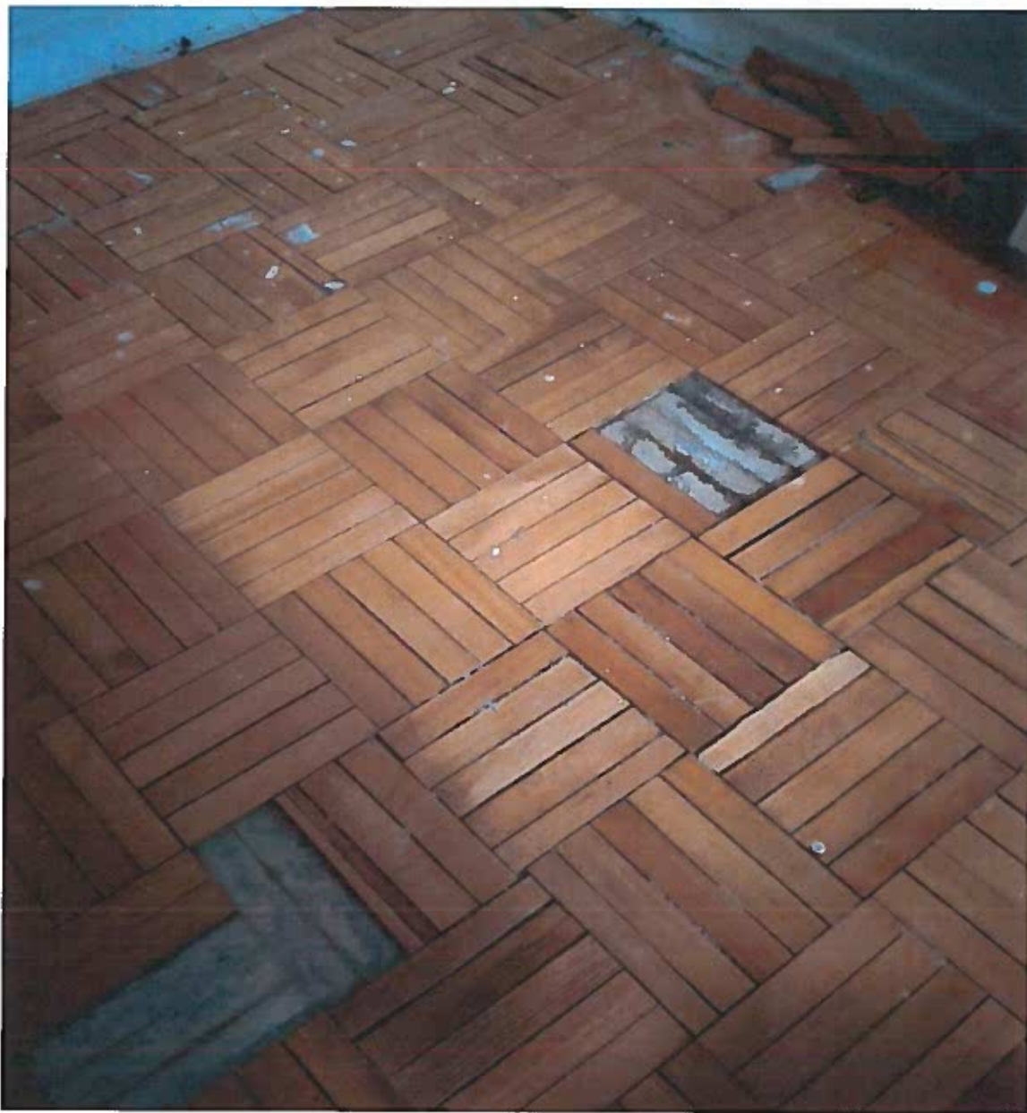
Item 3 – Broken and Missing Parquet Flooring
