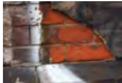
Damaged brick face under stucco
