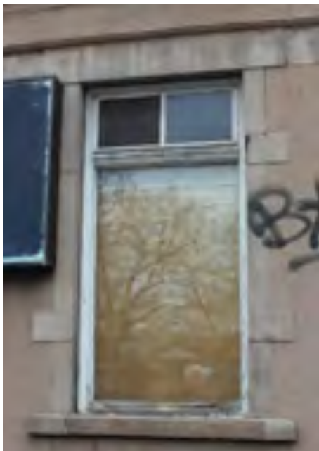
Typical original wood window frame along the front portion of the house. Note the stain glass transom
