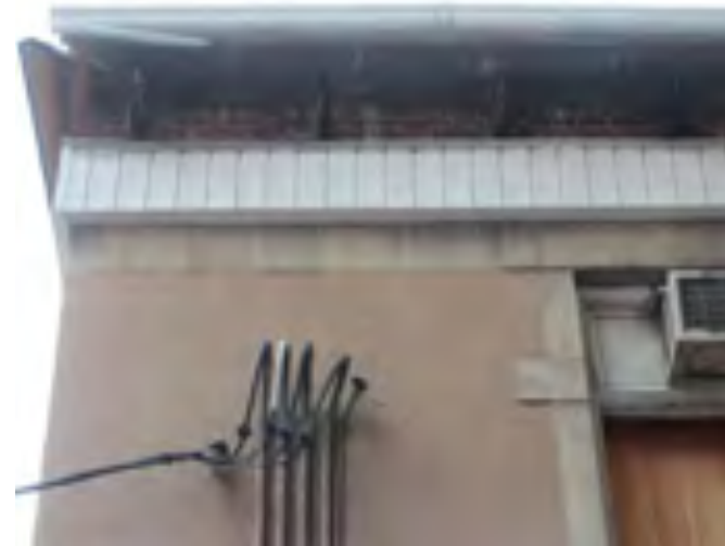
Burnt and damaged lookout rafters along the north facade. Temporary roof structure above.
