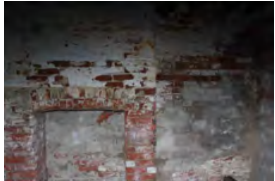
Masonry foundation wall along south facade. Note the parking, painted bricks, efflorescence buildup and fireplace
