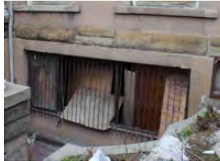
Modified basement window opening along the east facade. Note the two rock face stone lintels of the original openings.
