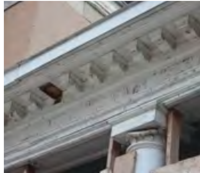
Front porch cornice. Note the flaking paint, missing bracket, improper replacement at column capital and metal flashing at top of the cornice
