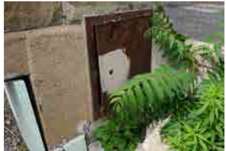
Image showing decommissioned electrical box to be removed and infilled with stone, note non-original stucco finish to the left of the electrical box (Source: GBCA, 2020)
