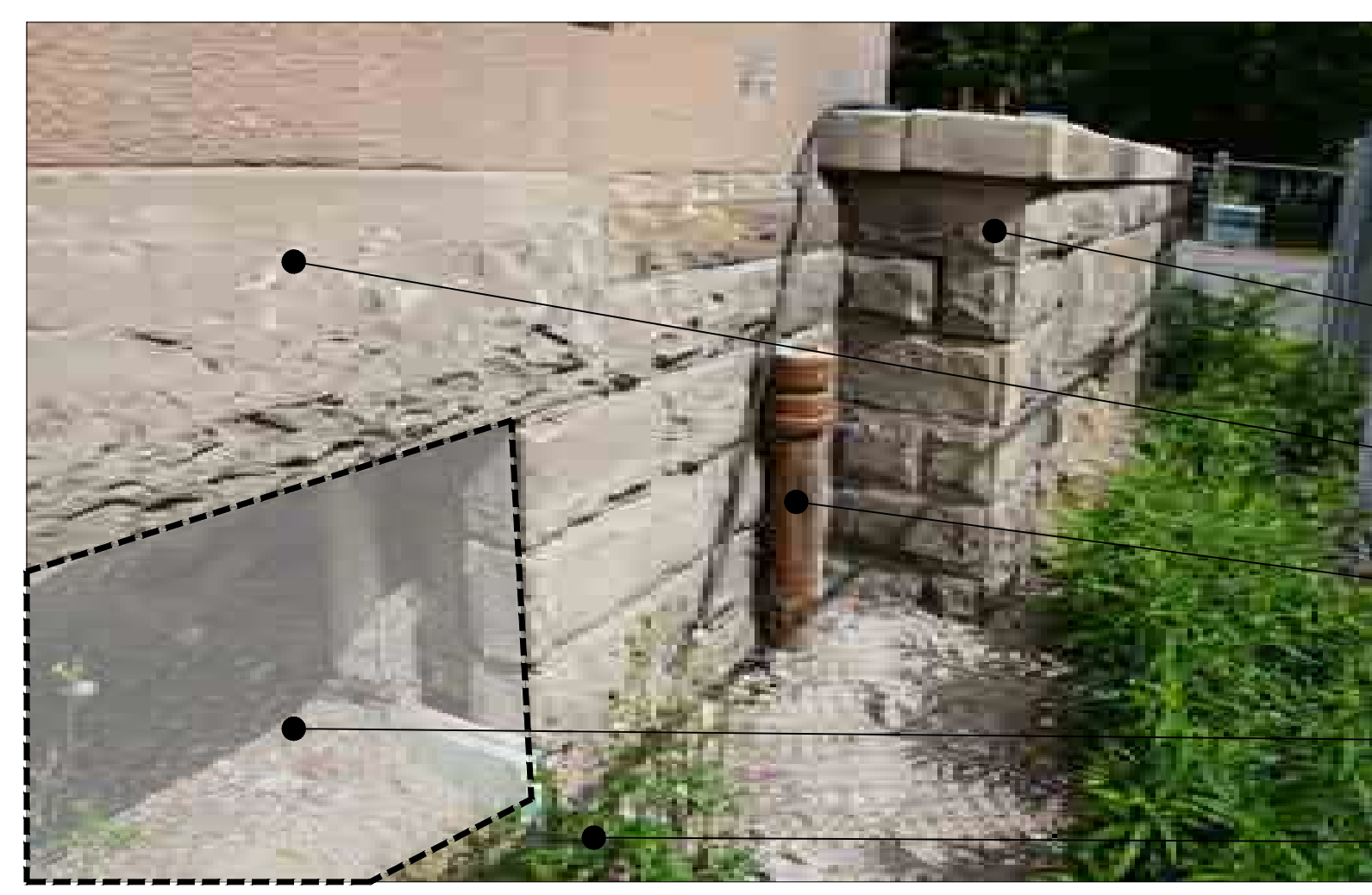
3 SOUTH ELEV. SOILING AND DETERIORATED RUBBLE STONE N.T.S
