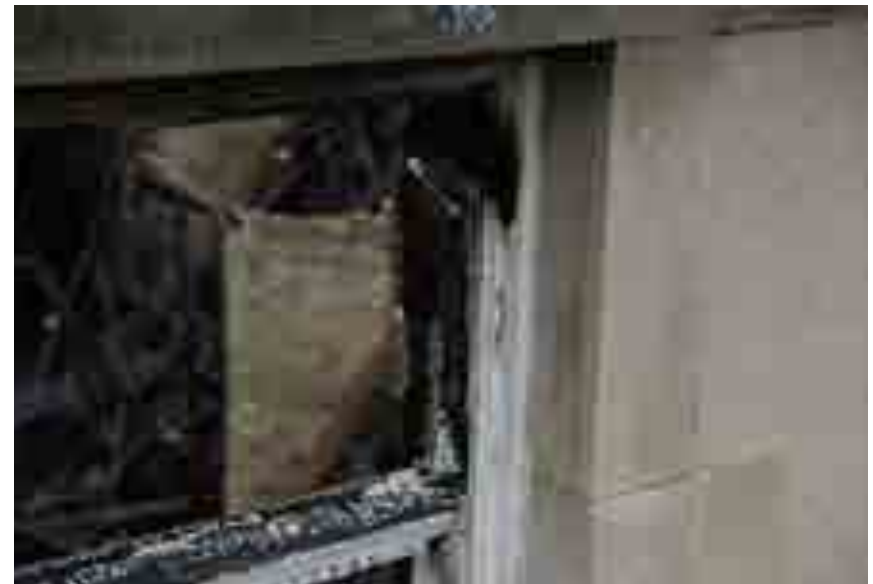
Detail showing destroyed wood window after 2019 fire (Source: GBCA)
