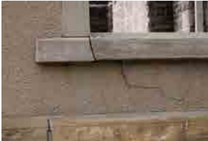
Detail showing cracked and displaced stone sill (Source: GBCA, 2020)
