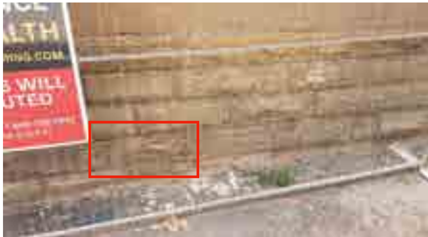
Image showing typical condition along north foundation wall, note deteriorated stones (red box) and efflorescence (Source: GBCA, 2020)
