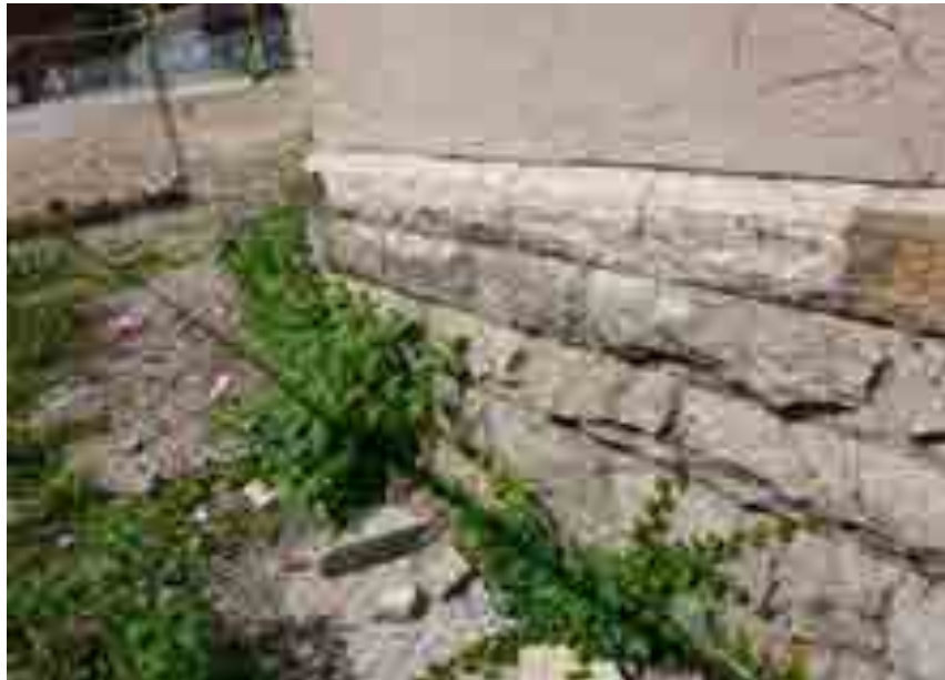
Image showing raised stone foundation with paint staining, biological growth and vines (Source: GBCA)
