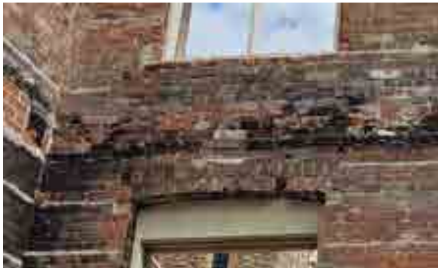
Interior detail showing damaged masonry arch at window opening, note deteriorated mortar joints and brick staining (Source: GBCA, 2020)
