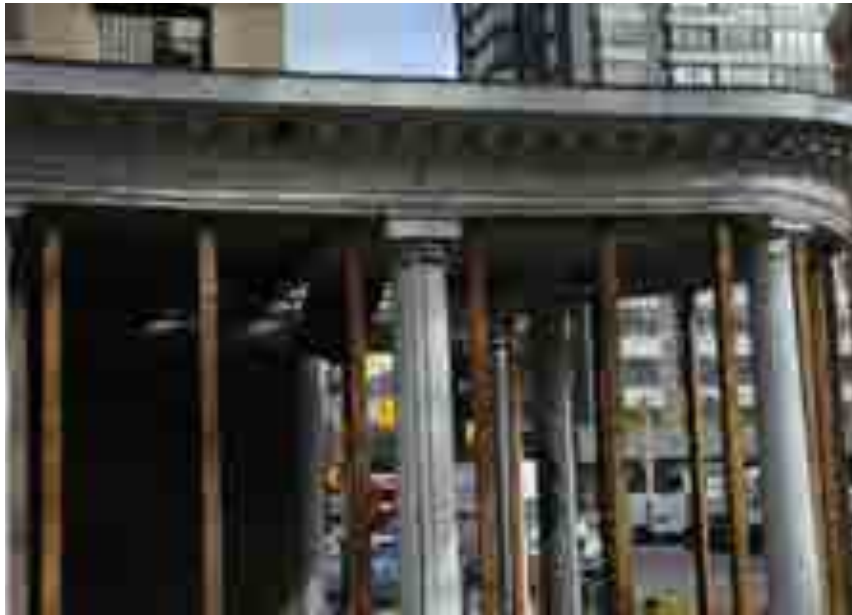
Image showing damaged wood porch after the 2019 fire (Source: GBCA, 2019)
