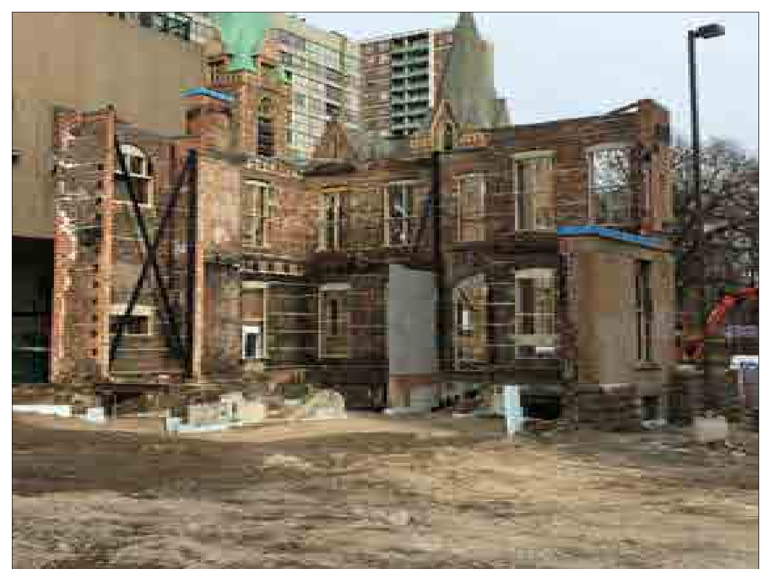
2 CURRENT SITE PHOTOS SHOWING CONDITION AFTER 2019 FIRE N.T.S.
