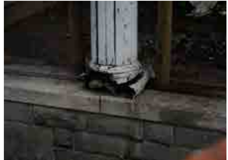
Detail Image showing damaged wood column (Source: GBCA)
