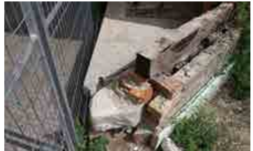
Detail showing northwest foundation wall segment and non-original curb to be removed (Source: GBCA, 2020)
