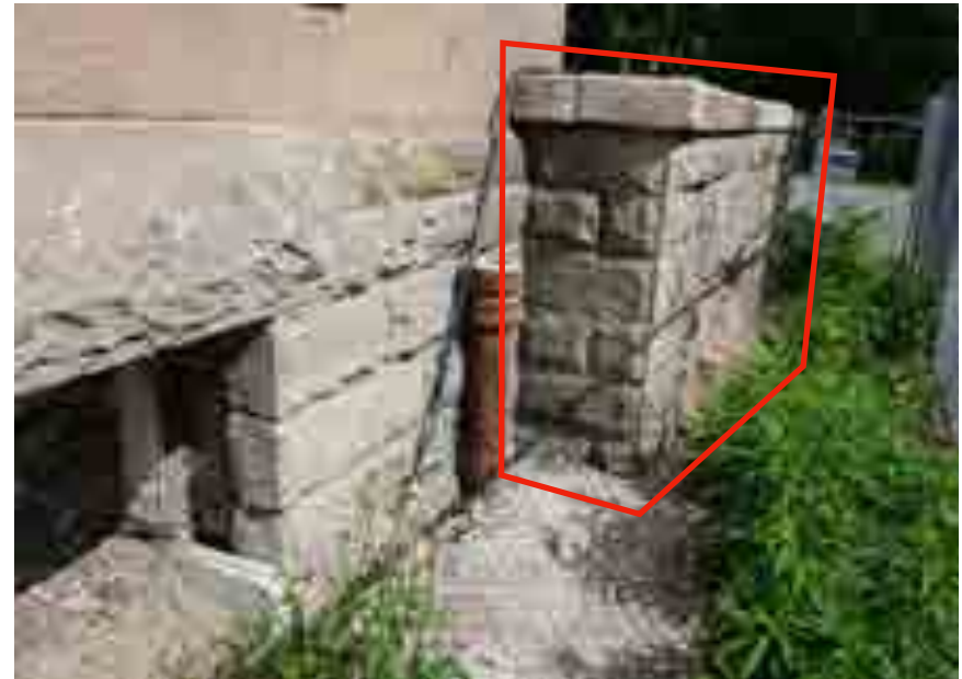
Image showing decommissioned opening to be infilled and efflorescence staining. Red box indicates portion of front porch stone base to be dismantled and reconstructed, refer to section '3.2 Front Porch' below for more information (Source: GBCA)
