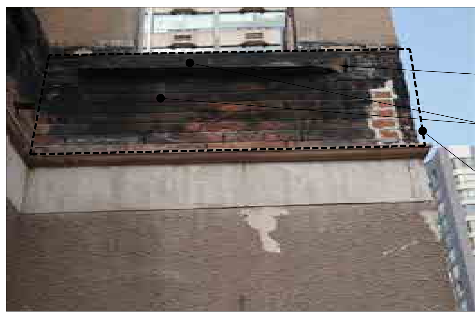
2 SOUTH ELEV. SOILING AND DETERIORATED WINDOW SILL N.T.S
