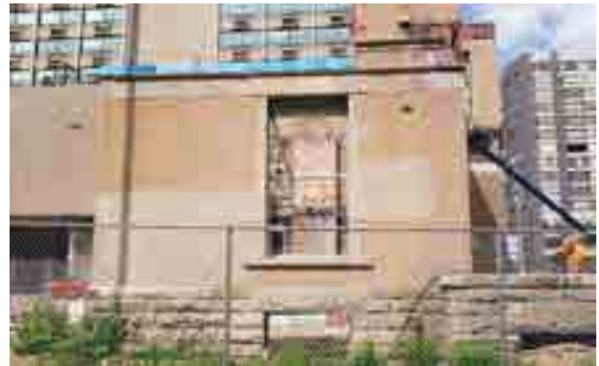
Image showing remaining south wall portion, note deteriorated stucco parging and staining at stone band course (Source: GBCA, 2020)
