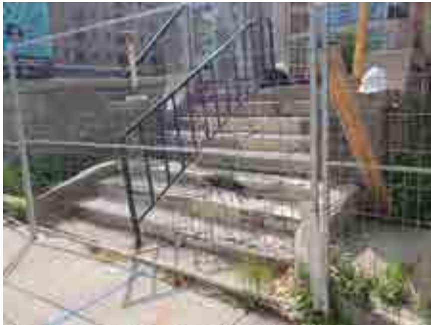
Image showing existing entrance steps condition, note deteriorated surface, exposed rebar, chipped ceramic tile finish and modern central handrail (Source: GBCA, 2020).
