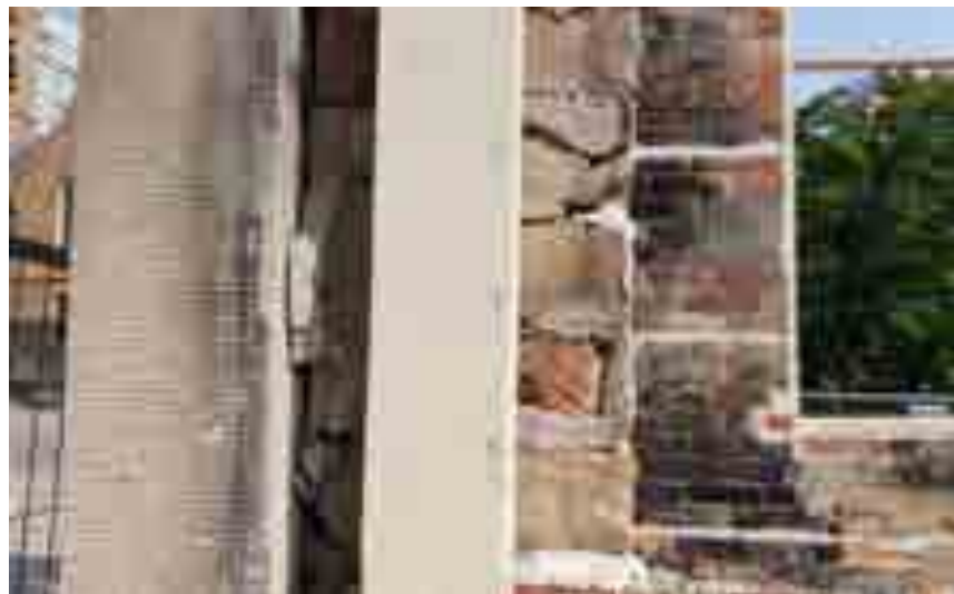
Image showing multi-wythe masonry wall at typical window opening, note staining at stone window surround (Source: GBCA, 2020)
