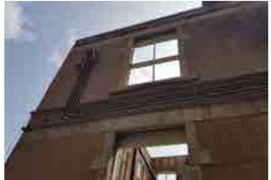
Image showing deteriorated stucco parging, stained stone band and decommissioned electrical conduits to be removed (Source: GBCA)
