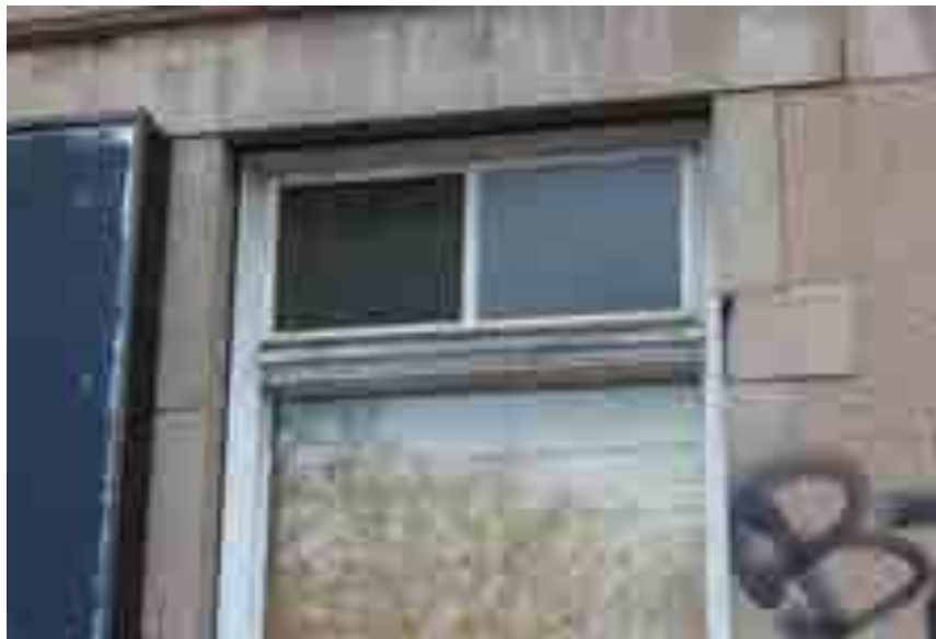
Image of typical east elevation wood window showing condition before 2019 fire (Source: GBCA)
