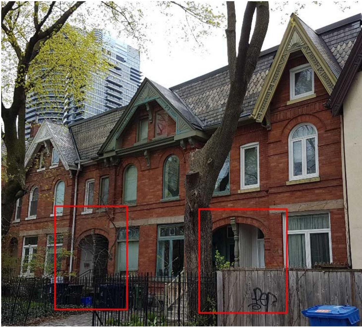
Image 12. Current photograph showing the type of original, shared, round-arched entryways of the heritage properties at 76-84 McGill Street typical of the neighbourhood and that existed at 79 and 81 Granby Street prior to their alteration. (Heritage Planning, 2021)
