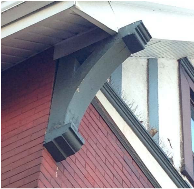
9. 685 Queen Street East: Photograph showing the detail of the decorative profiles of one of two brackets supporting the projecting overhang of the roof. (HP, 2015)
