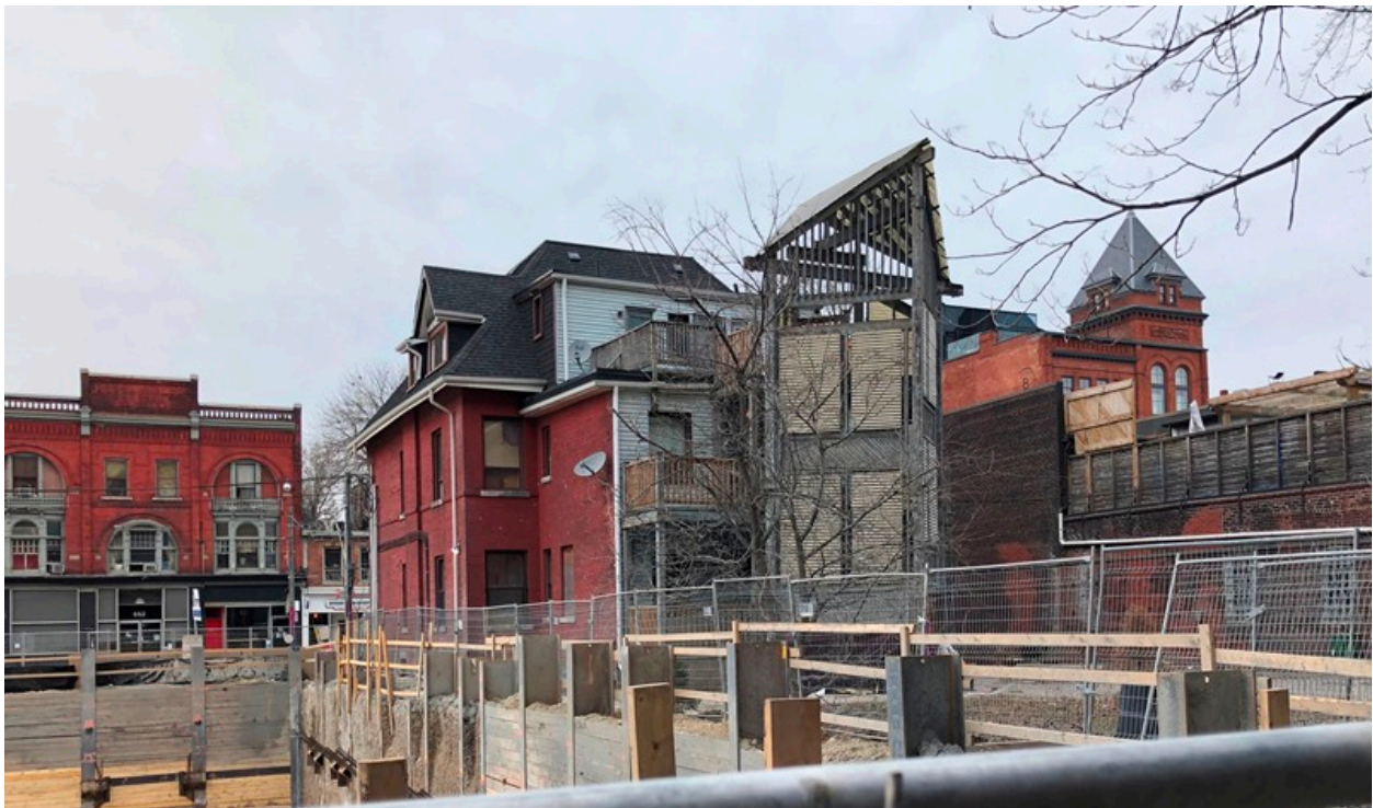
12. 685 Queen Street East, south and west elevations with rear wing: photograph showing the south side of the house with the rear, lower wing and the modern addition of a screened fire escape. (HP, 2021)
