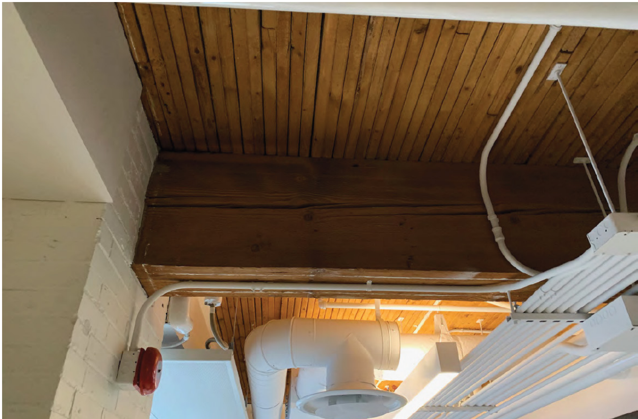
Detailed view of the interior heavy timber post and beam structure of the front (east) portion of 906 Yonge Street (ERA Architects Inc., 2021)
