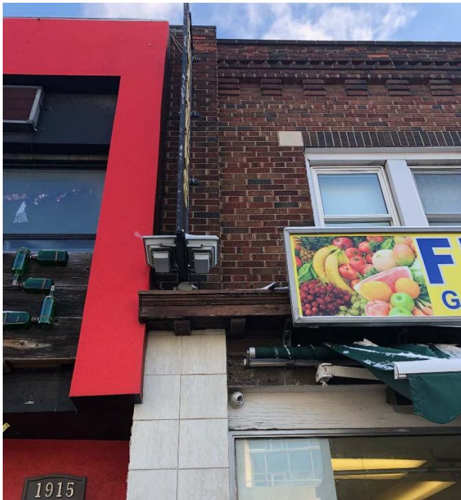
16. Photograph showing the dentilated wooden cornice and brick and stone details above the storefront on 1913 Yonge Street's west elevation. (Heritage Planning, 2021)
