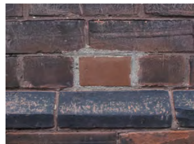
Typical unsympathetic brick unit replacement and mortar repair (ERA, 2018).
