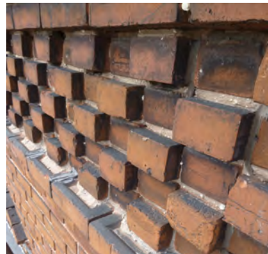
Decorative string course of checker-board pattern bricks; cement mortar repair (ERA, 2015).
