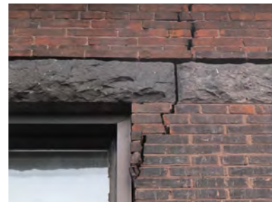
Significant masonry step cracking on south facade (ERA, 2018).
