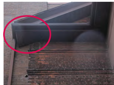
Peeling soffit at the north elevation. (ERA, 2018).
