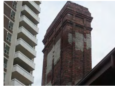
Unsympathetic parging repairs on chimney (ERA, 2015).
