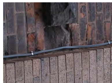
Stone detailing has been removed (ERA, 2018).
