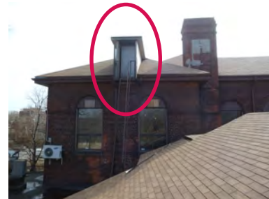
West elevation of the roof on heritage building with new dormer outlined (ERA, 2015).
