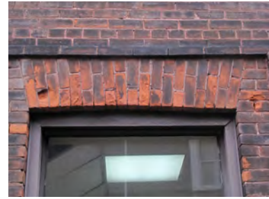
Typical brick spalling on arch detailing above window (ERA, 2018).
