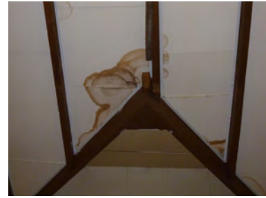
Water damage visible in attic (ERA, 2015).
