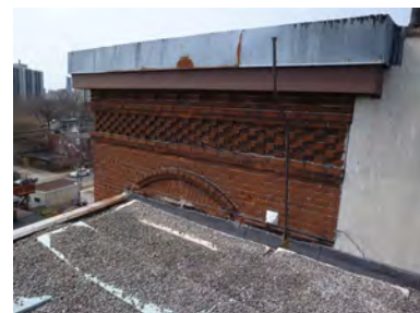
Rusted metal flashing on tower (ERA, 2018).
