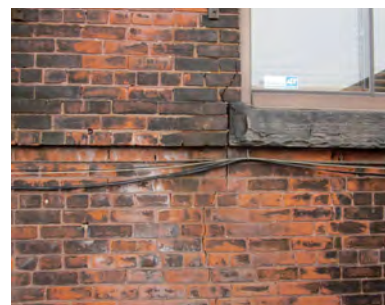
Minor cracking, typical soiling, and wires attached to the west elevation (ERA, 2015).
