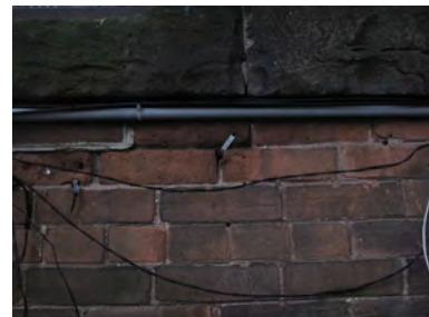
Obsolete anchors and wires on north facade. (ERA, 2018).
