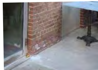
Efflorescence at east entrance (ERA, 2015).
