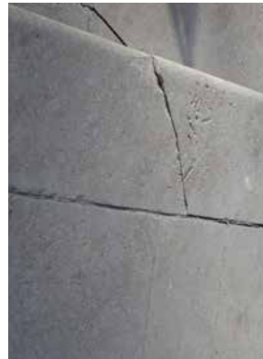
Cracked stone steps at south entrance (ERA, 2015).
