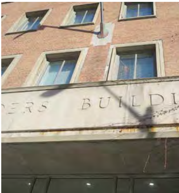
Stains on stone masonry at main entrance (ERA, 2015).
