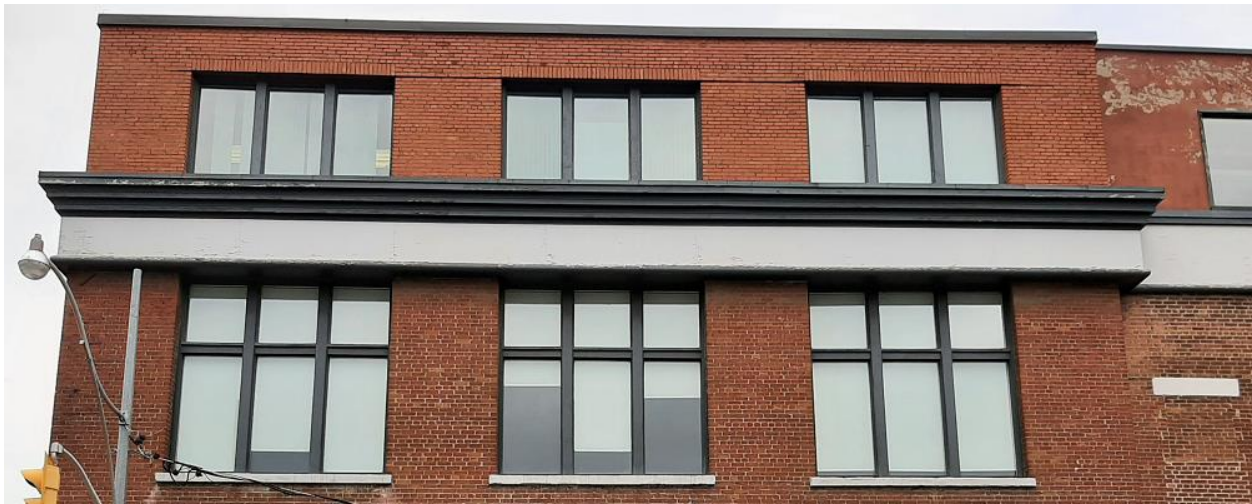
Image 22. Cornice detail upon the front (east) elevation of the former New Method Laundry building (today part of 544 and 550 Queen Street East). Heritage Planning, 2022.
