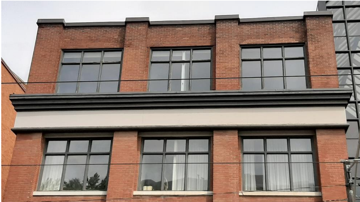
Image 18. Cornice detail upon the former National Electric Heating building (today part of 544 and 550 Queen Street East). Heritage Planning, 2022.
