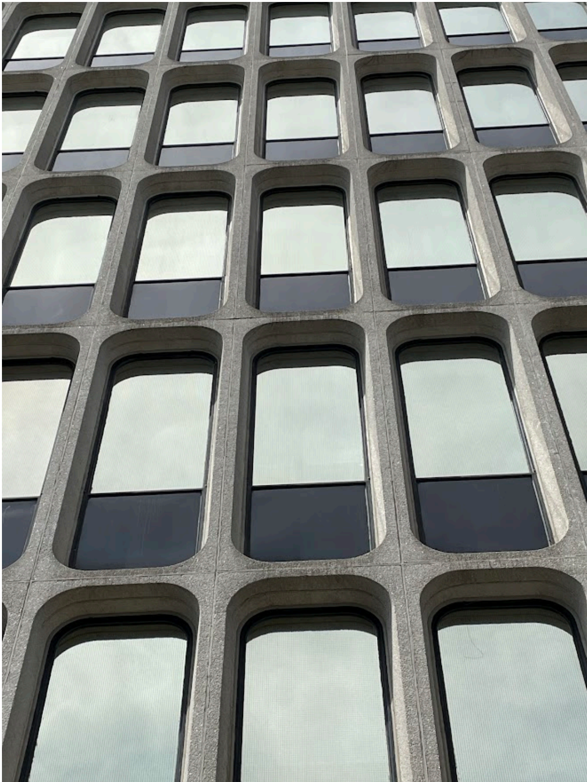
Image 16. Current photograph showing detail of the precast concrete panels and window openings (Heritage Planning, 2022)
