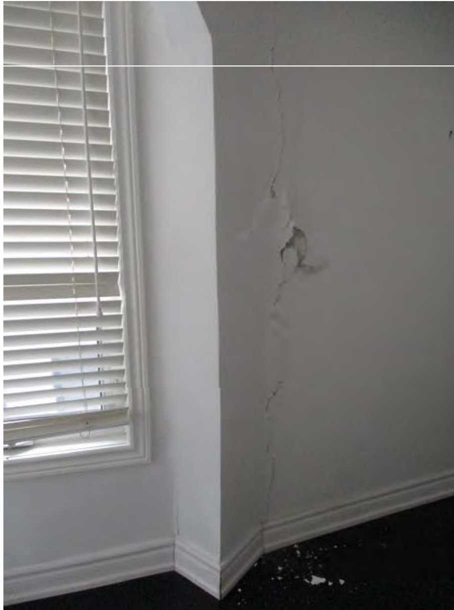
Photograph of the damaged east wall from the inside of the existing building at 12-14 Bishop Street.
