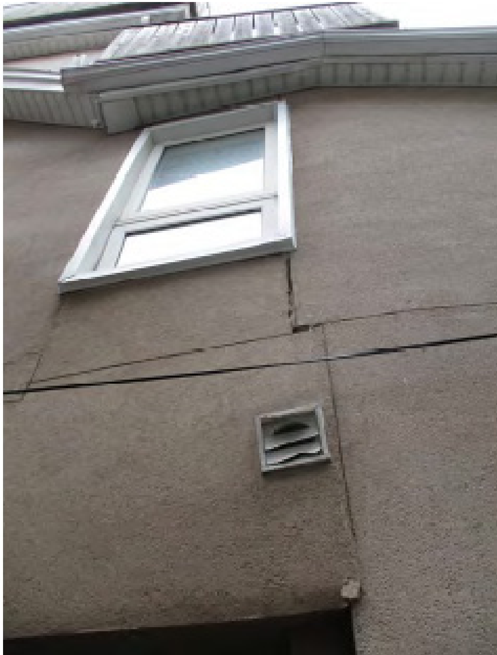
Photograph of the damaged east wall of the existing building at 12-14 Bishop Street.
