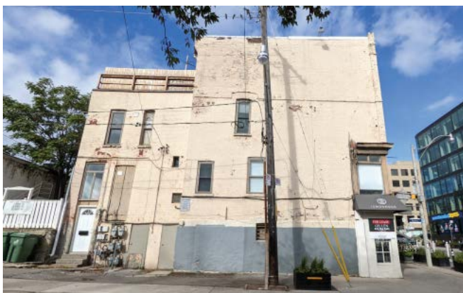
Image 19. 2021 Image of the south elevation of the corner property at 1196 Yonge (including 2 Birch Avenue) and showing the alterations to openings in the 1920s and a floating doorway at left that serves as a reminder of the earlier street grade.
