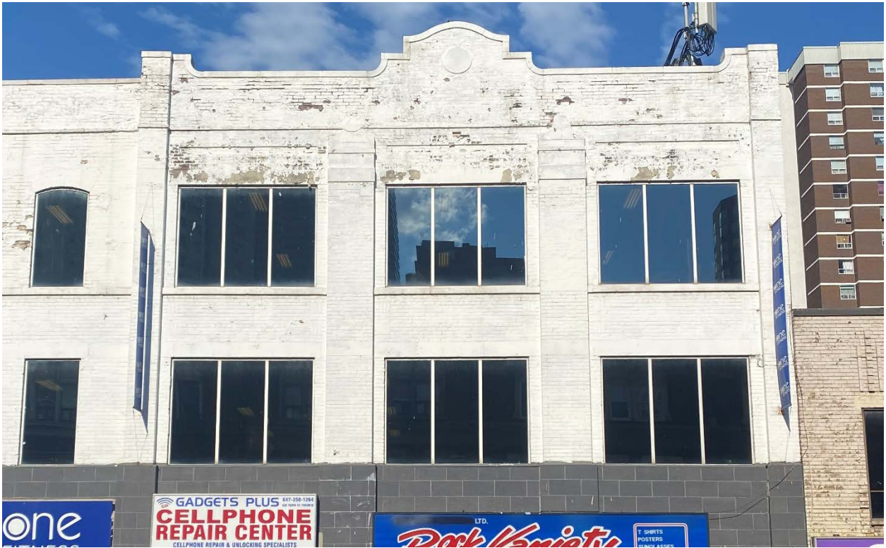
Figure 15: Detail of the west elevation of the southern building (625-629 Yonge Street), showing the brick parapet (Heritage Planning, 2022).
