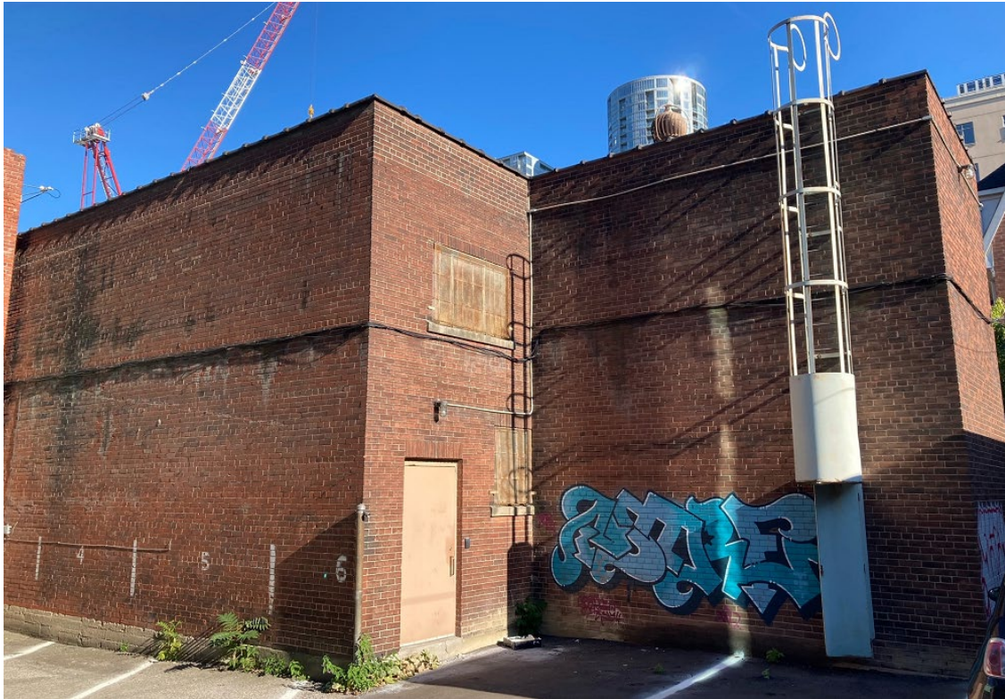
Image 14. 18 Portland Street. Side (north) and rear (east) elevations. Note the metal replacement door. Heritage Planning, 2022.
