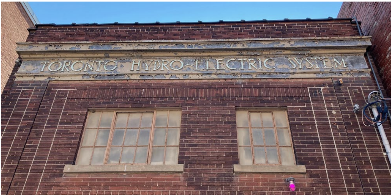
Image 12. Close-up view of 18 Portland Street. Note the metal entablature with sign band, factory type windows, brick masonry details, and terracotta coping. Heritage Planning, 2022.
