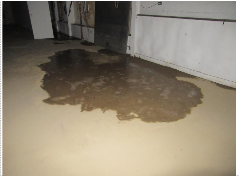
PHOTO NUMBER 7: Slab on grade NOTE: Ice present on slab on grade from flooding.
