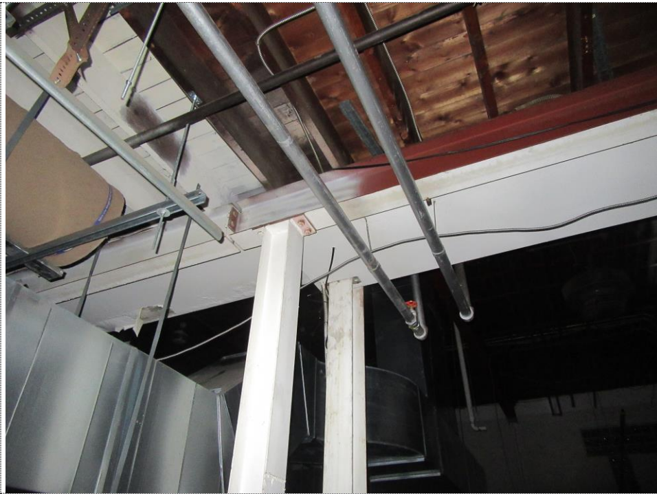
PHOTO NUMBER 5: Underside of west portion of roof structure. NOTE: Wood joists and wood decking
