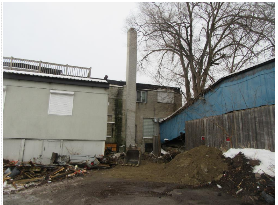
PHOTO NUMBER 2: Rear (east face) of building and abandoned covered walkway.
