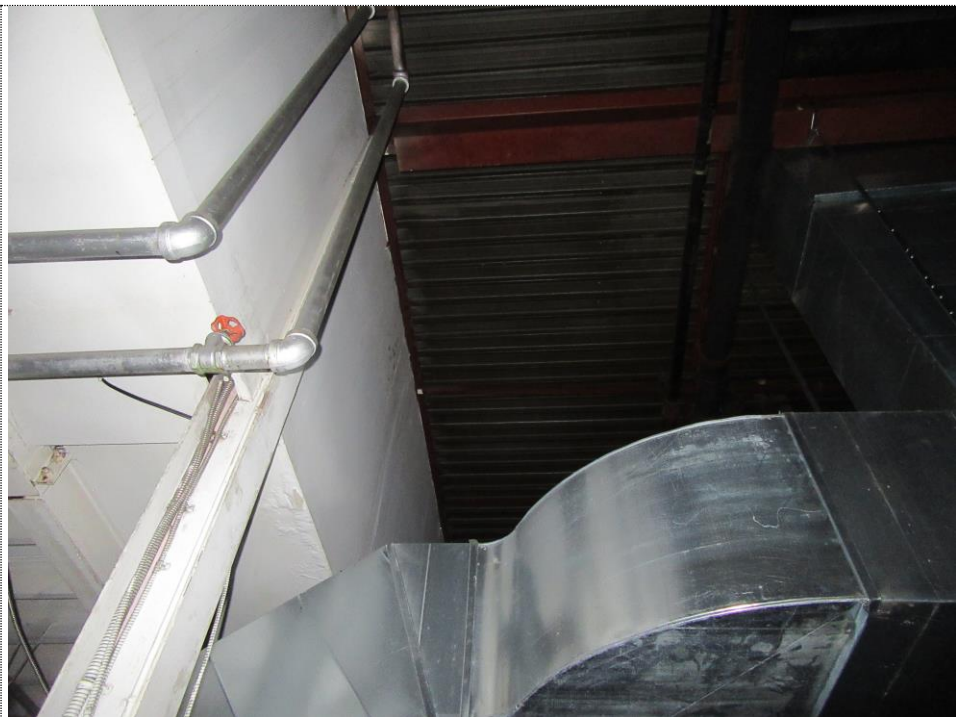
PHOTO NUMBER 6: Underside of east portion of roof structure. NOTE: Open web steel joists and metal decking
