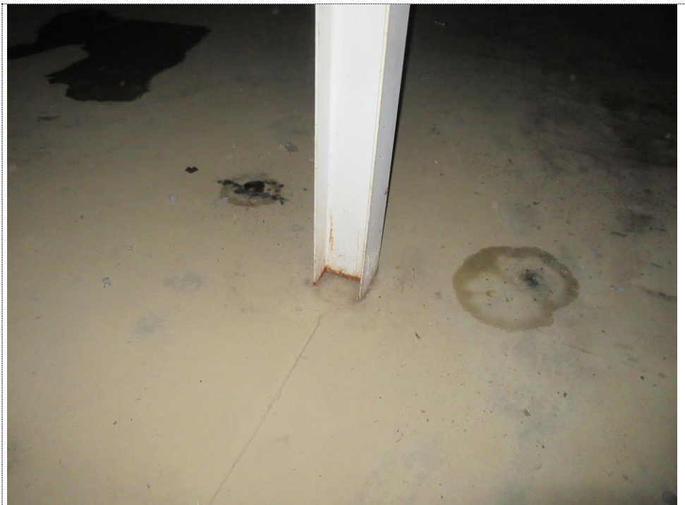
PHOTO NUMBER 8: Building interior column at slab on grade. NOTE: Corrosion of base of column.
