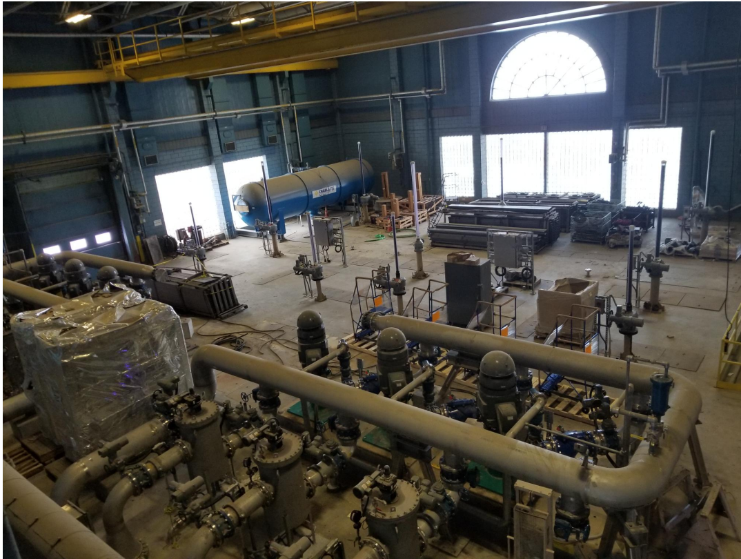
Figure 5 – Plant Water Pumping Station
