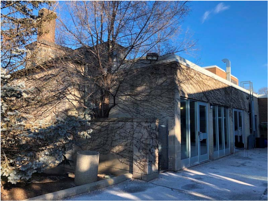
6. West and south elevations of the garage building with the extension of the ground floor to accommodate the school dining hall
