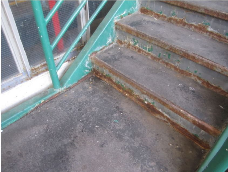
Figure 3: CP68 (20 St. Andrew Street) – Stairwell Photos No.3 Corrosion at stair treads and risers.
